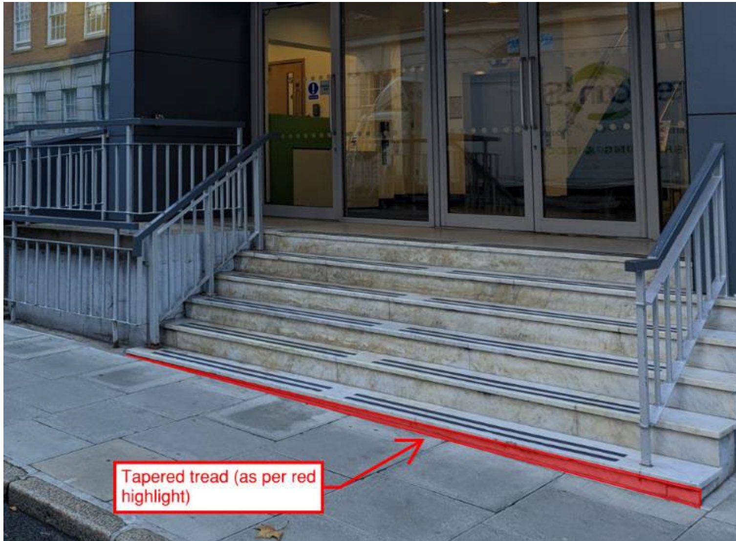
Figure 13. Photo showing the tapered tread, at the bottom of the main entrance.
