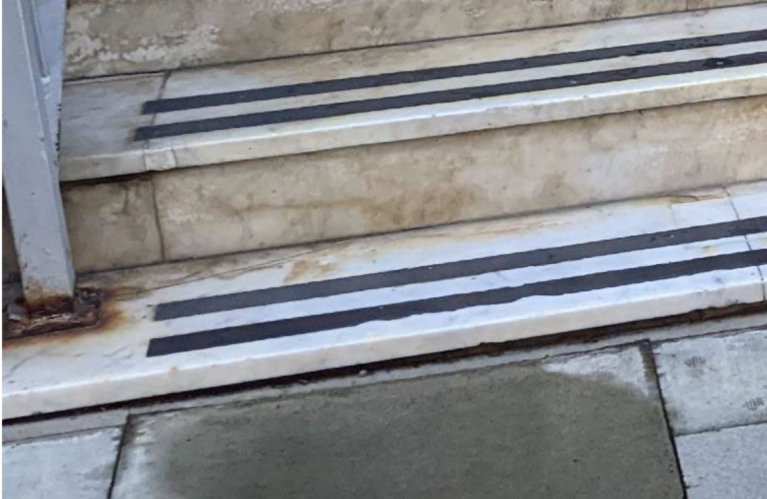
Figure 9. Detail of the stair nosing deterioration.
