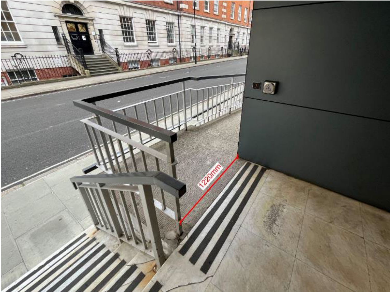
Figure 2. Indication of the current clear width of the top landing of the ramp (in red).
