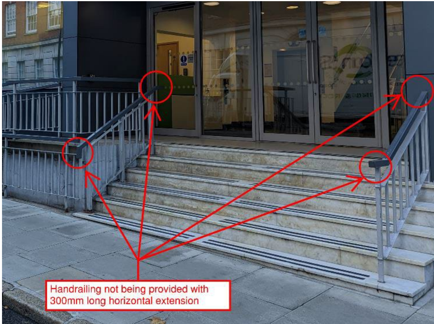
Figure 12. Photo showing lack of 300mm long horizontal extension to the stair handrails.
