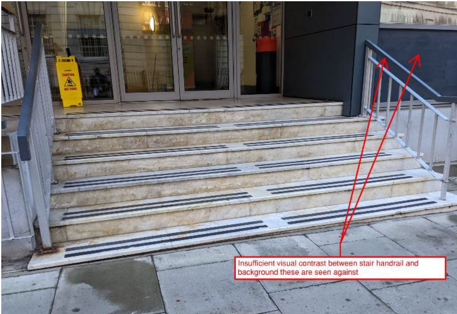
Figure 10. Photo showing lack of sufficient visual contrast between handrails and background these are seen against.
