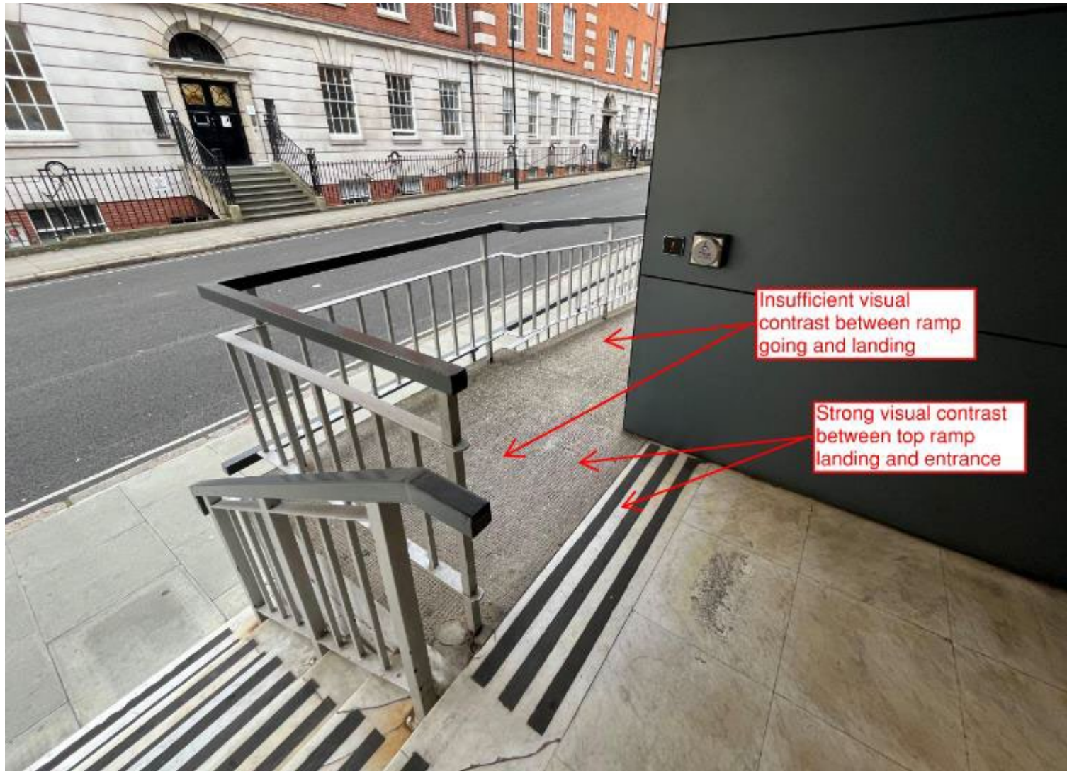
Figure 5. Photo showing lack of sufficient visual contrast between the ramp going and the top landing, in addition of strong visual contrast in the intersection between top ramp landing and entrance.
