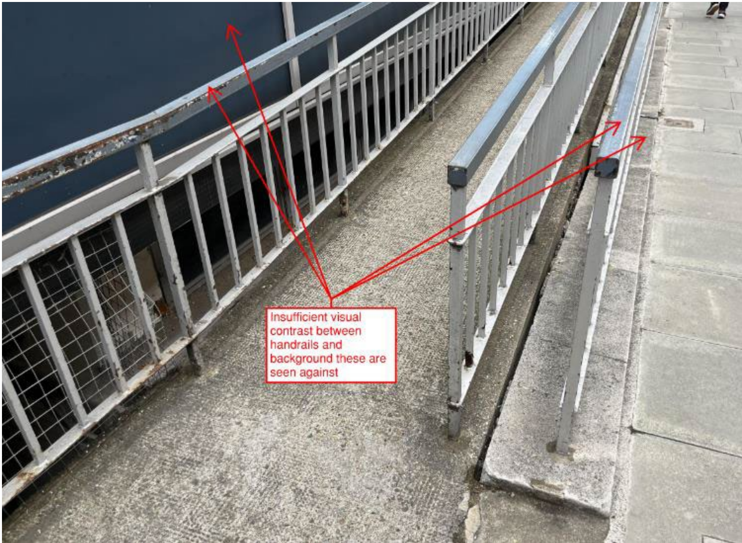
Figure 6. Photo showing lack of sufficient visual contrast between handrails and background these are seen against.
