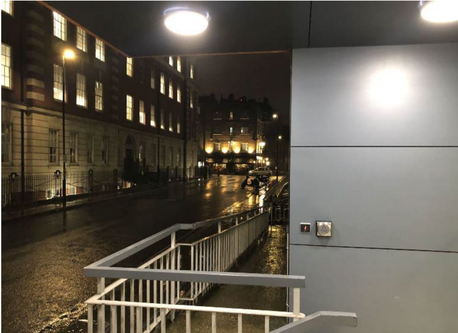
Figure 8. Photo showing the lack of sufficient illumination, along the ramp, during nighttime conditions.
