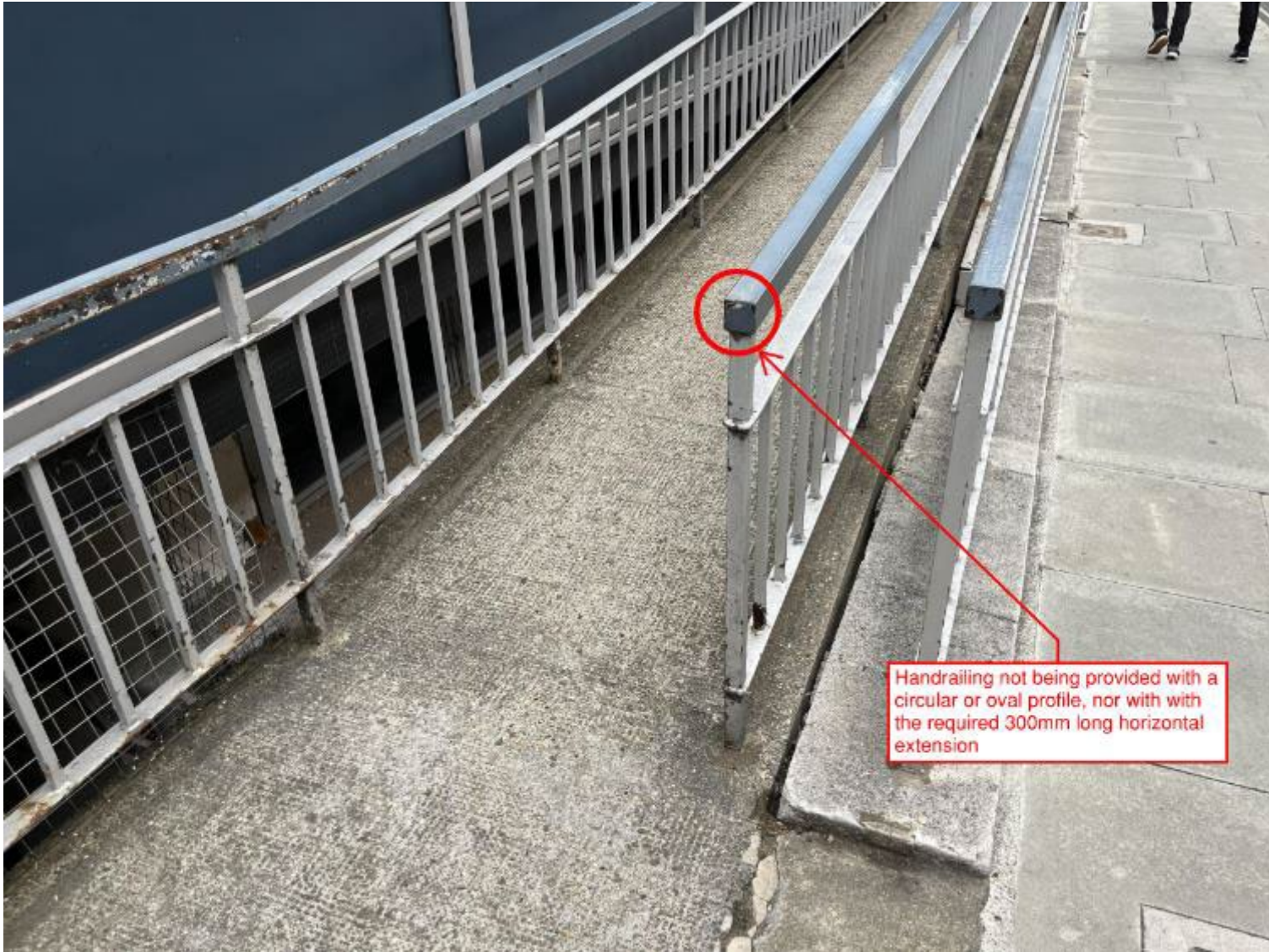
Figure 7. Photo showing lack of circular or oval handrailing profile, and lack of 300mm long handrail horizontal extension.
