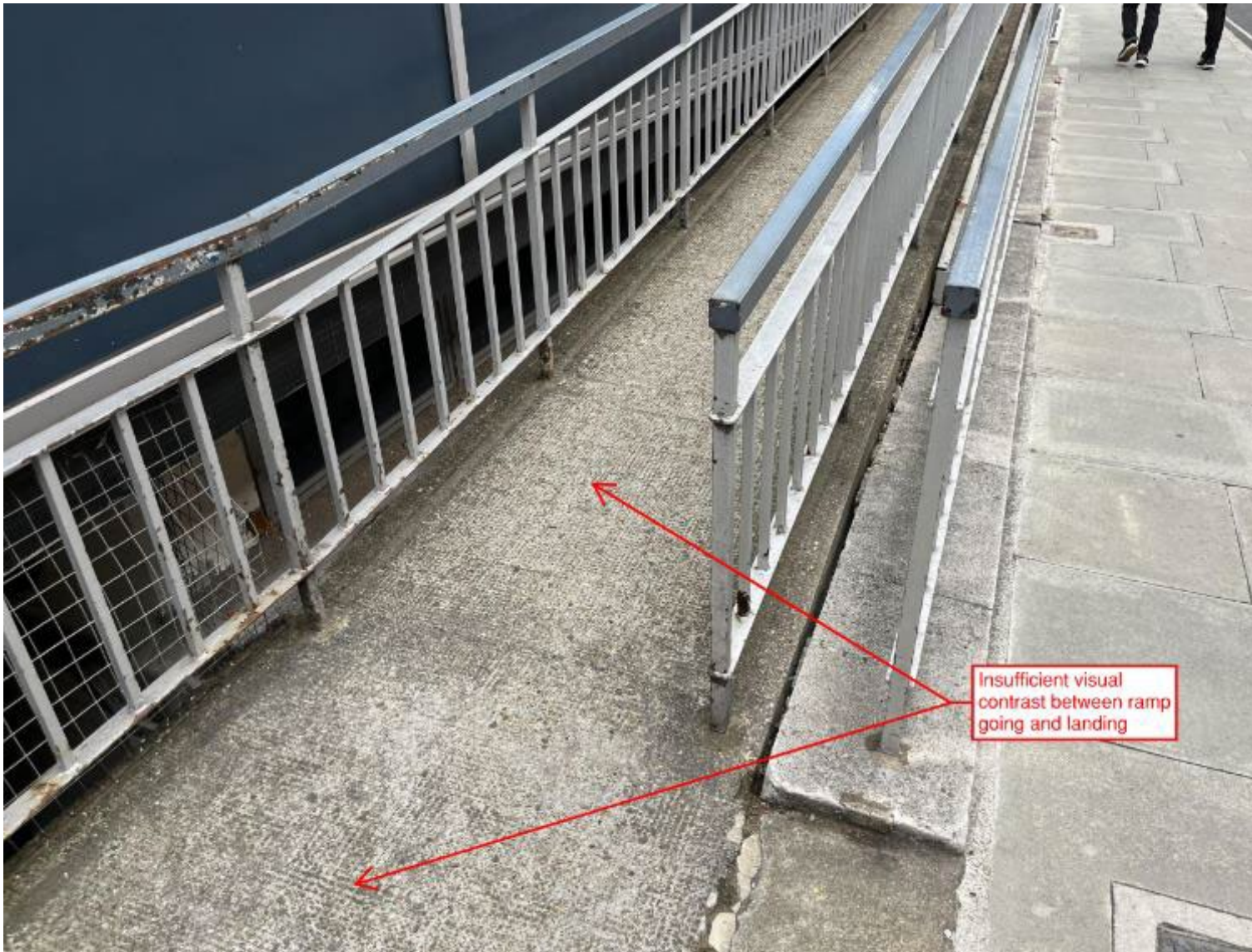
Figure 4. Photo showing lack of sufficient visual contrast between the ramp going and the bottom landing.
