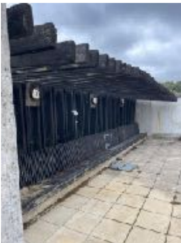
Timber loggia on the roof requiring repair/replacement as necessary.
