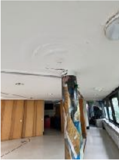
Ceiling Damage in Hall and Floor damage
