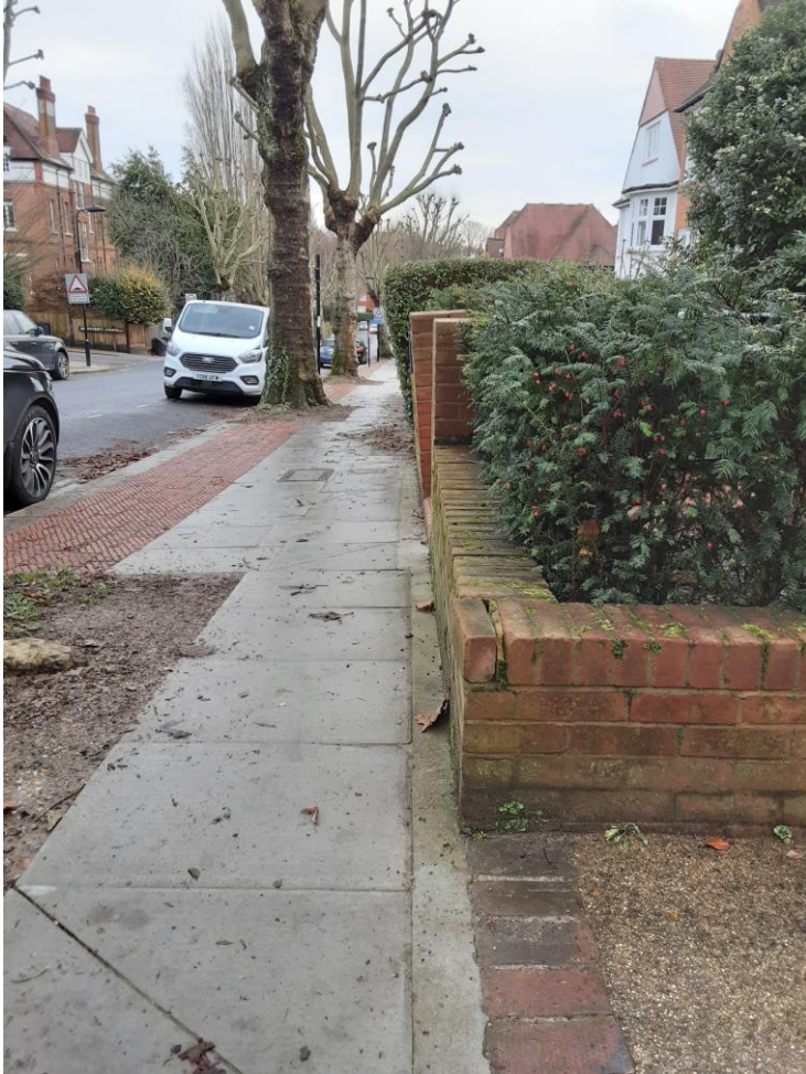
Photo 3: Brick pillar leaning towards pavement
