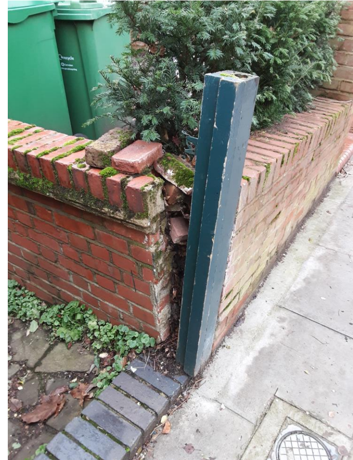
Photo 2: Damage to neighbours gate post and wall
