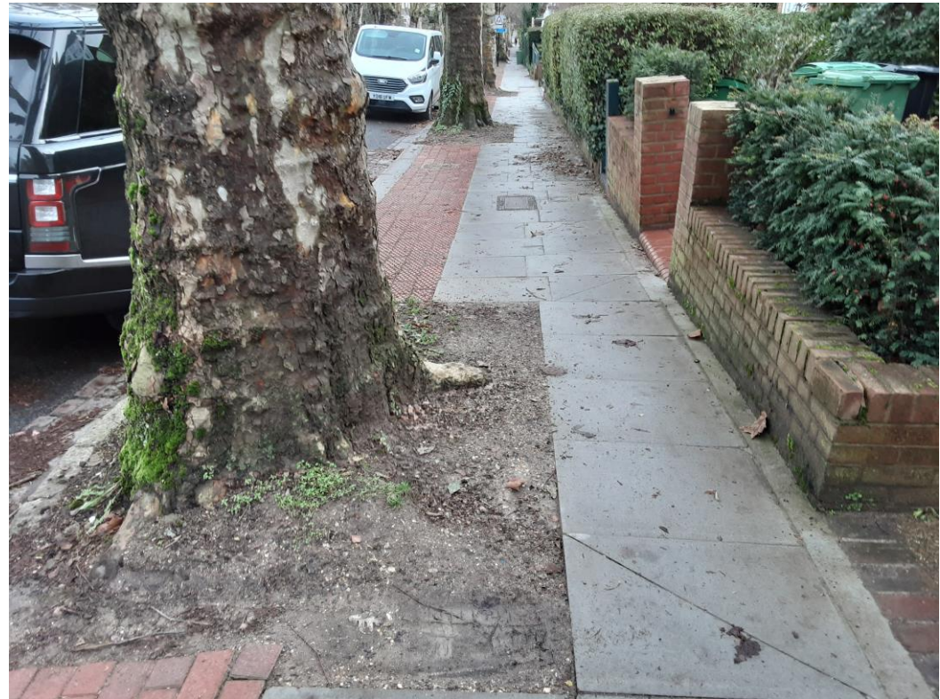
Photo 4: Damage to wall corner and brick pillar in relation to tree
