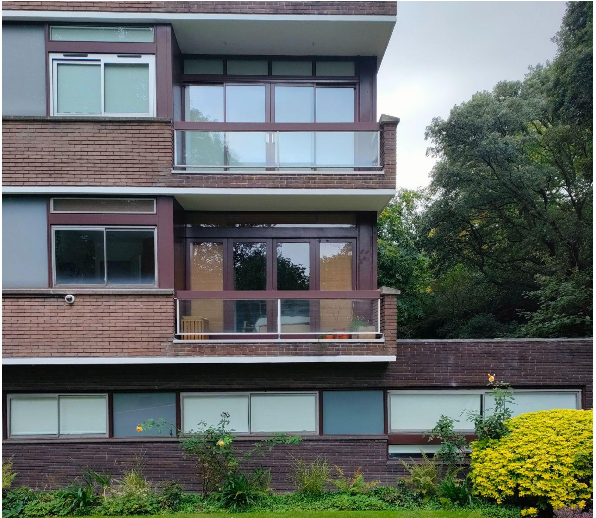
Image 9. Existing balcony doors below and aluminum frames of neighbours above.
