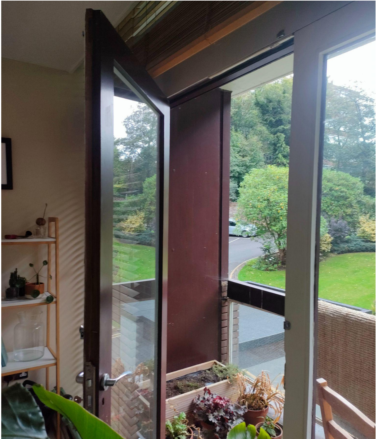
Image 8. Existing (fragile) lock mechanism and external colour of the balcony doors, to be maintained.
