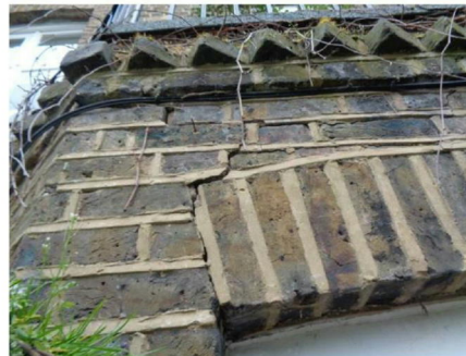
Cracking where the arch has failed
