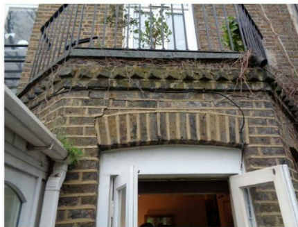
The damaged arch over the French doors in the single storey rear bay
