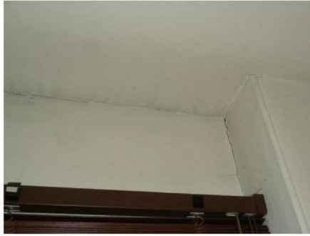
Cracking in the living room over the rear bay reveal
