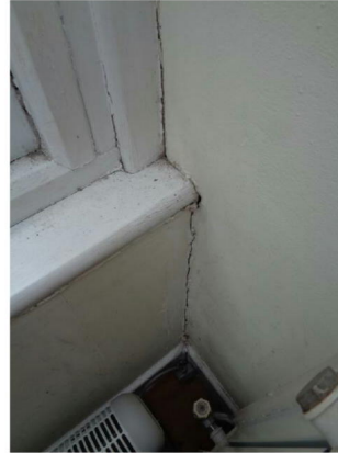
Crack at the right side of the conservatory at the junction with the main building
