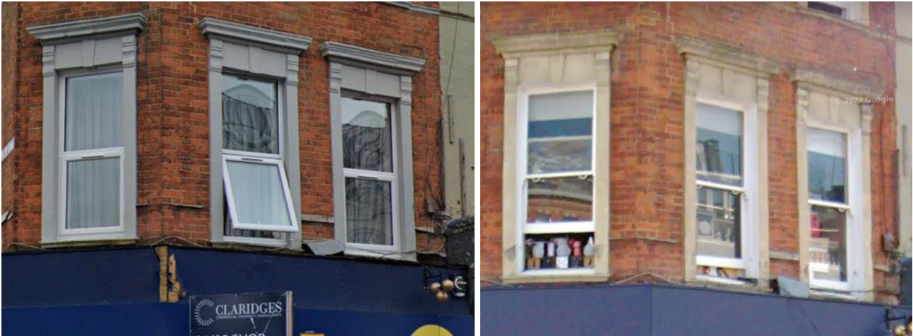
Figure 1 – [Left] New unauthorised uPVC window opened. [Right] Prior timber sash windows opened.
