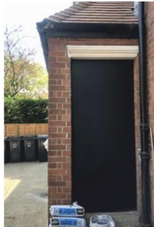
C. Existing blocked door in flank wall to be removed and bricked up in bricks to match existing
