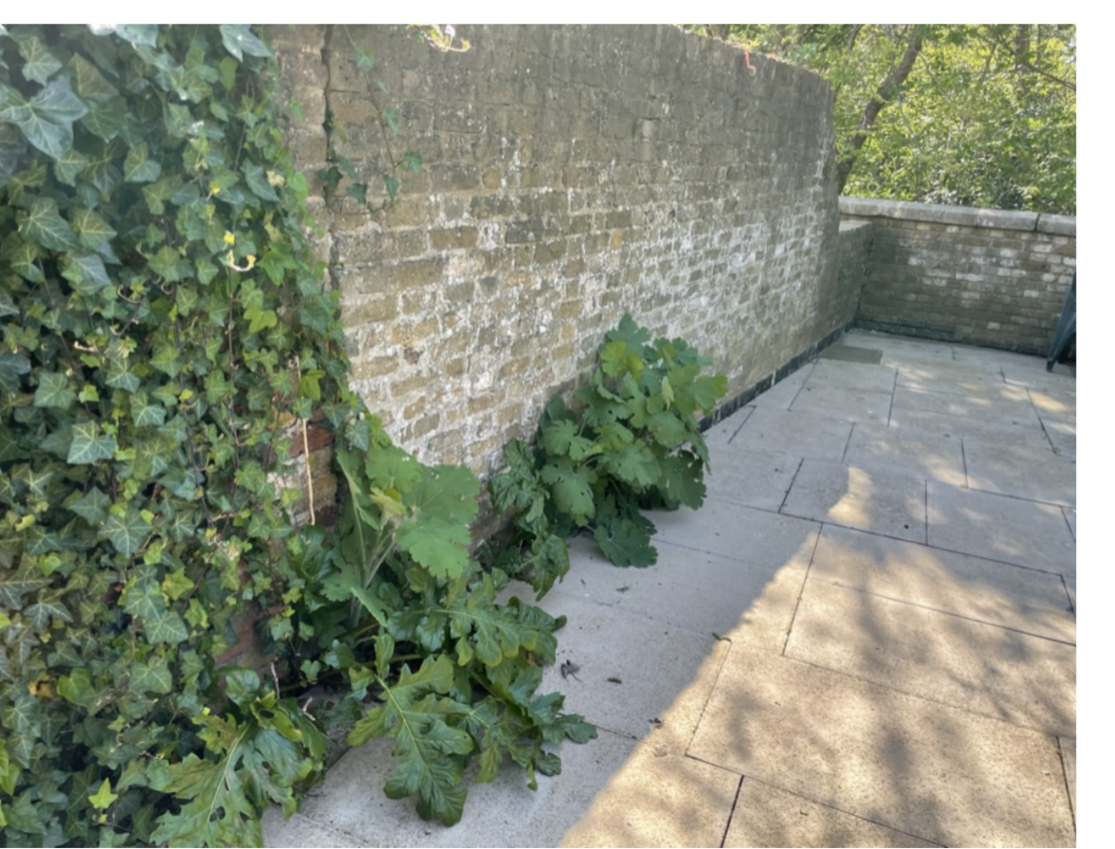
PHOTO 5: REAR WALL TO HIGHGATE CEMETERY ABOUTING NEIGHBOURING WALL LOOKING SOUTH EAST TO 103 SWAIN'S LANE NOT TO SCALE
