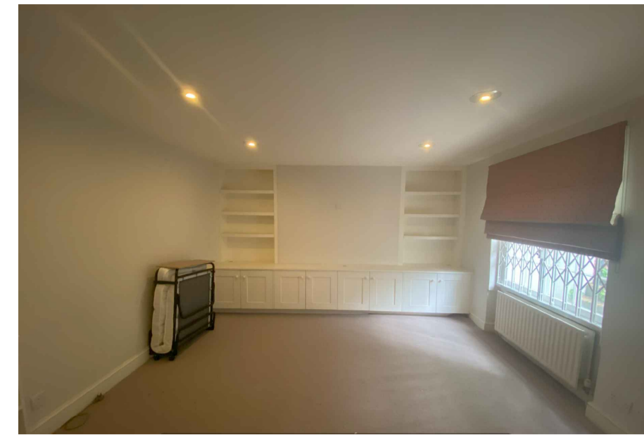
1 Lower Ground Front Room - Ceiling To Be Replaced image SCALE 1: na
