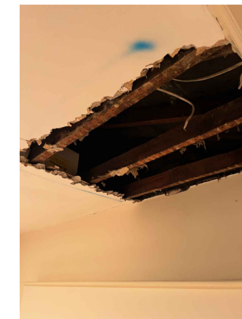
2 Damaged Plasterboard Ceiling In Loft image SCALE 1: na
