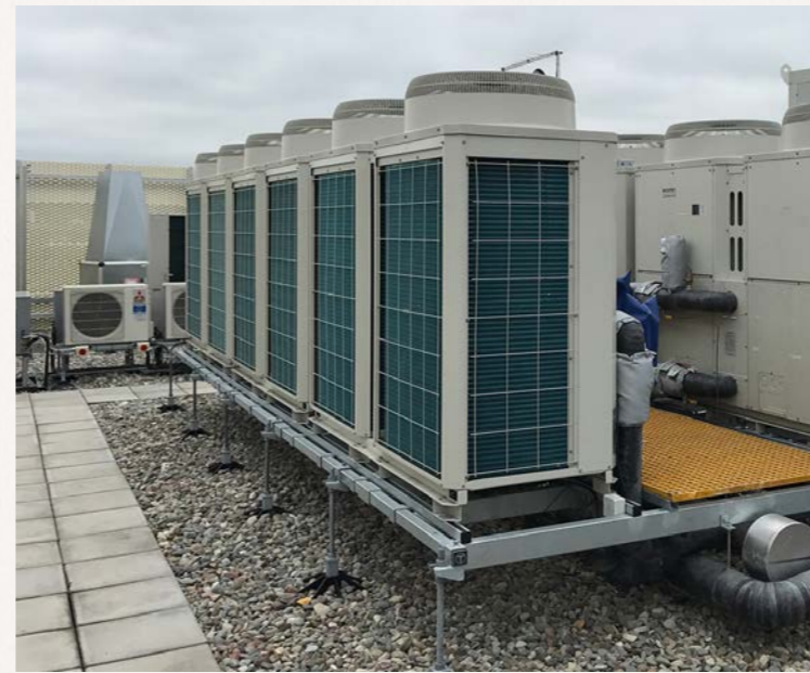
Air Source Heat Pumps
