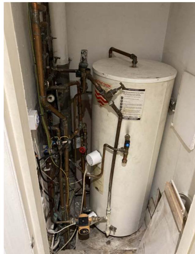
Fig. 53. 1st floor boiler room
