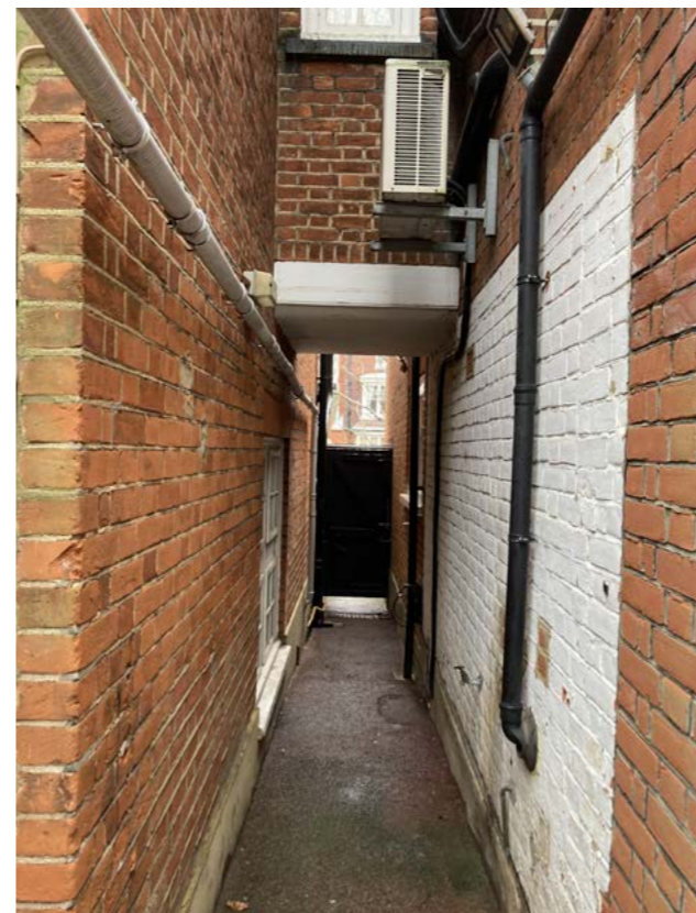
Fig. 62. Right of way passage between no 26A and 26 and 1st floor link
