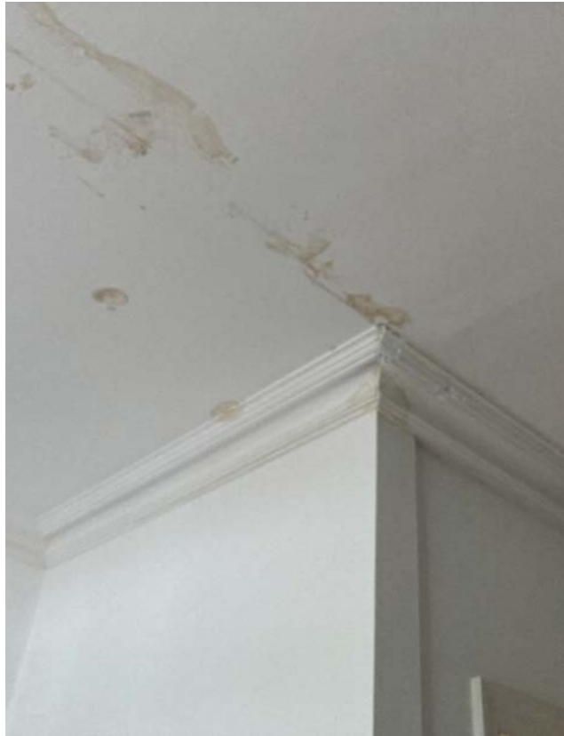
Fig. 50. 1st floor ceiling - water damage
