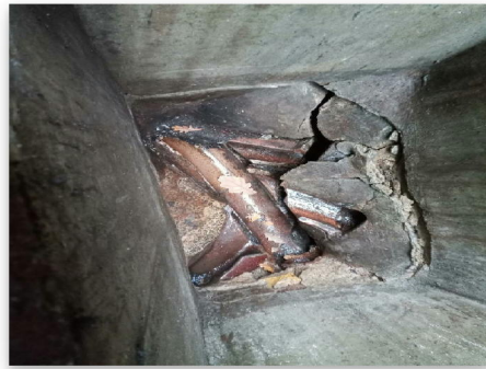
Fig 3.2: Defective manhole channel/ benching
