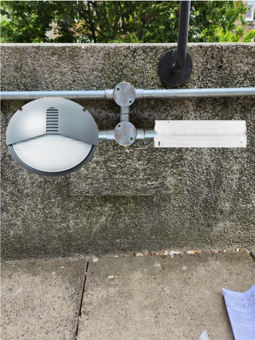
5.2 Site Location – Proposed Photo Level 5 – With emergency luminaire arrangement
