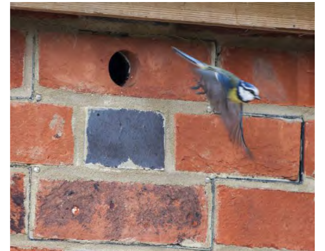
Integrated bat & bird boxes in facades to increase biodiversity
