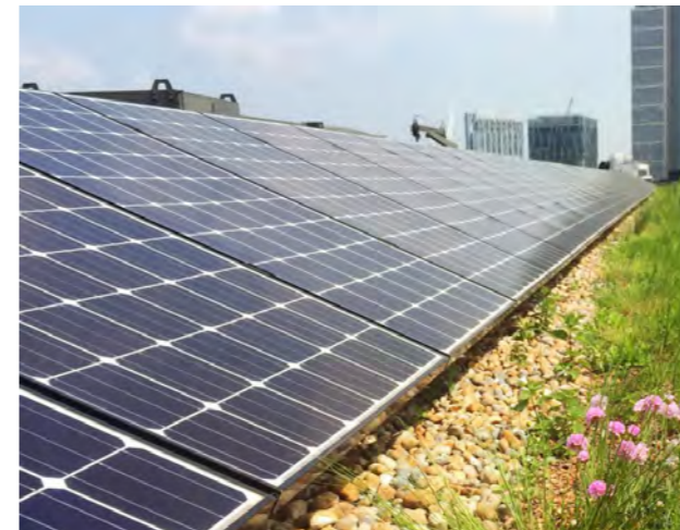
PV panels at roof level
