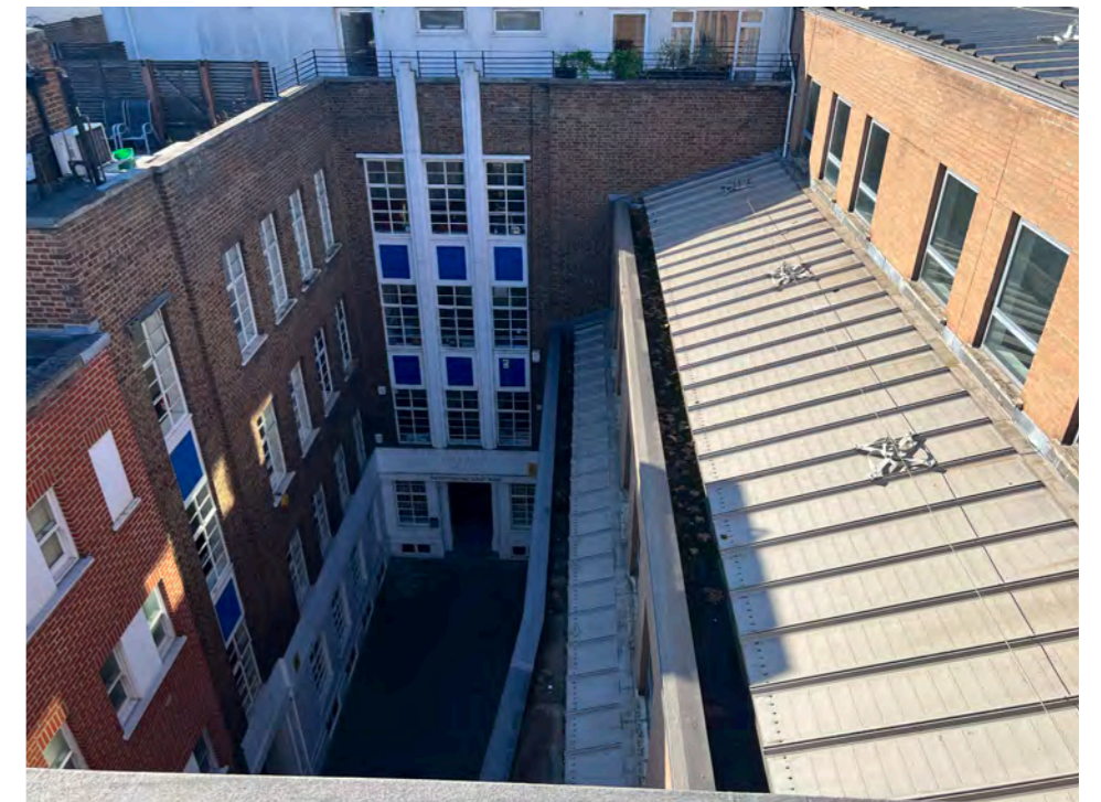
View of the existing metal roof to be reconfigured into a roof terrace
