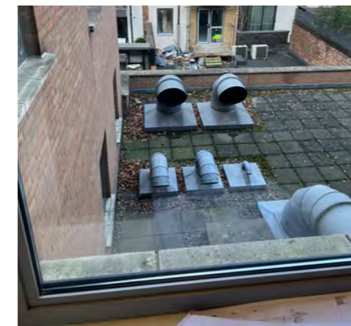
Existing roof plant at 1st floor
