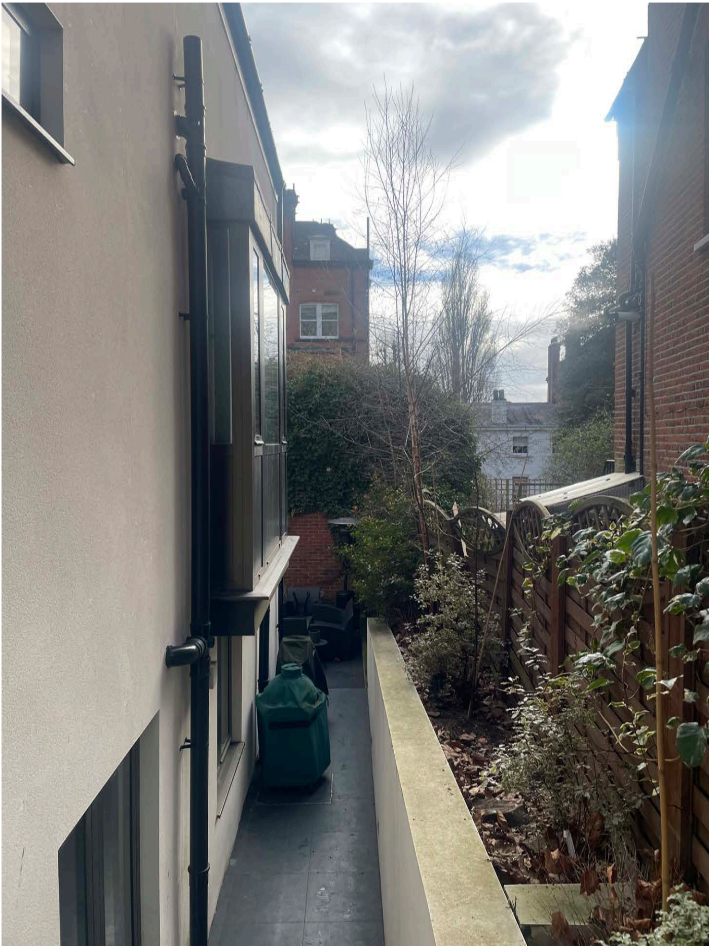
The Existing Fence is rotting and has collapsed. It has been temporarily propped to keep it upright.
