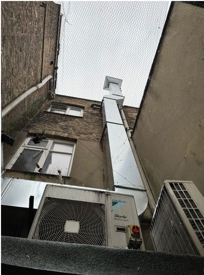
Photo 1 View of exhaust ductwork from yard
