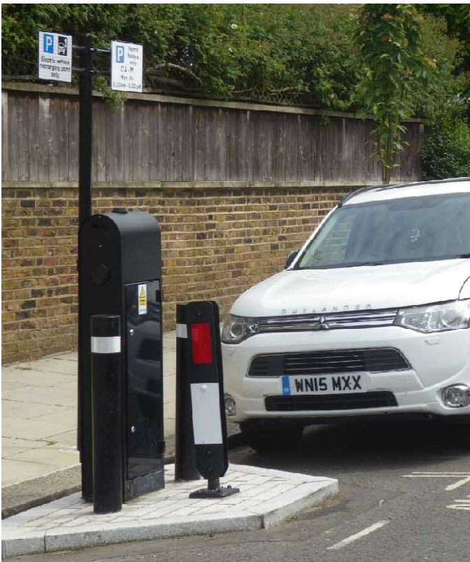
Figure 8 Photo showing electric car charging point on Ospringe Road.
