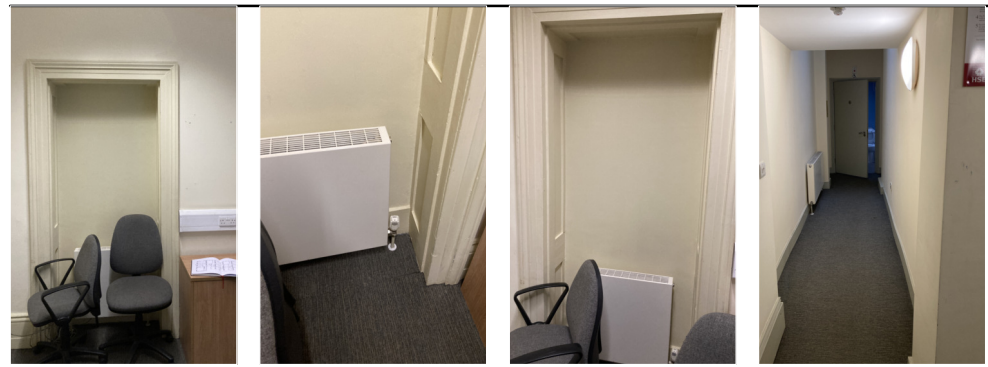
EXISTING INFILLED DOOR (ROOM SIDE) EXISTING INFILLED DOOR AT LOW LEVEL (ROOM SIDE) EXISTING INFILLED DOOR (ROOM SIDE) INFILLED DOOR - DECORATED IN (CORRIDOR SIDE)
