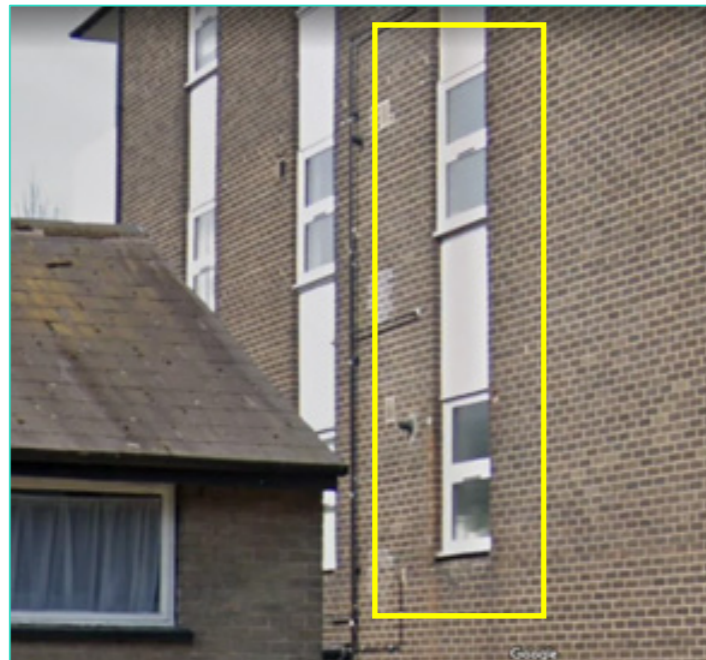
Drawing Extract 02: photo demonstrating probable bathrooms or WCs. Windows W4/101 (first floor) and W4/102 (second floor) highlighted yellow
