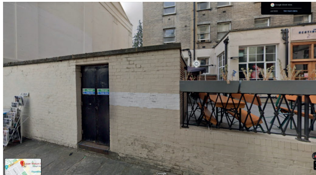
Fig. 13. Existing substation ©Google Street View 2023
