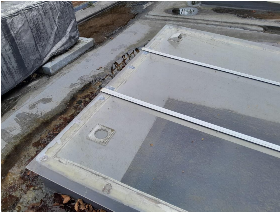
Photograph 7: Opening in skylight providing potential access point (Target Note 3, Figure 1)
