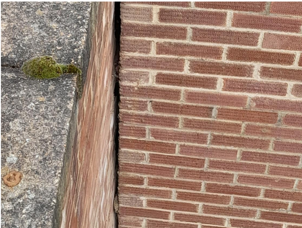
Photograph 6: Wall crevice leading to a cavity space (Target Note 1, Figure 1)
