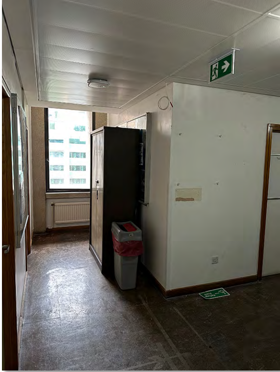
IMG_7295 Corridor area between Rm 350 & Rm 352 showing wall where proposed new door is to be installed
