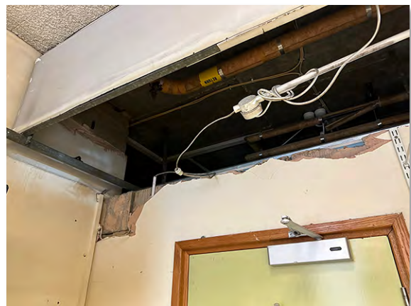
IMG_7255 Rm 249 ceiling bulkhead – later addition blockwork sits below bulkhead soffit
