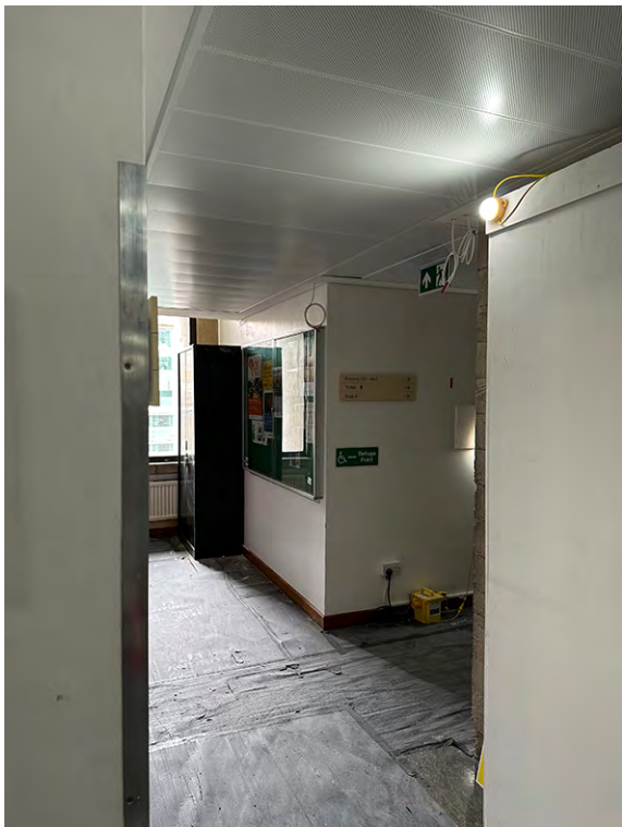
IMG_7318 Corridor area between Rm 400 & Rm 401 showing wall where proposed new door is to be installed
