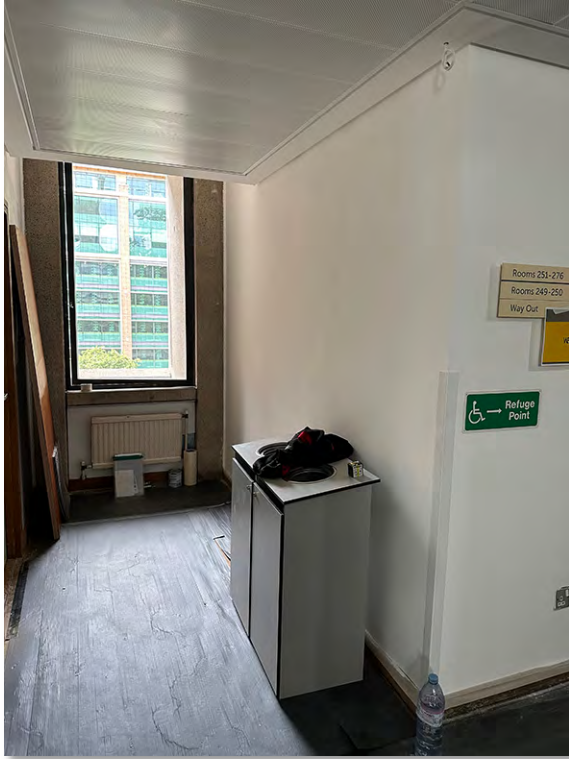
IMG_7281 Corridor area between Rm 250 & Rm 251 showing wall where proposed new door is to be installed
