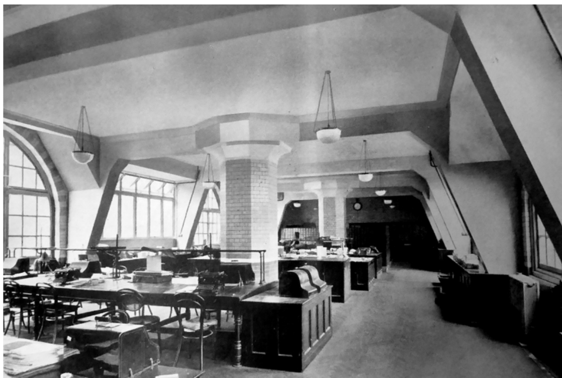
Figure 9: Views inside the raised attic floors showing reinforced framing that also supported the new flat roofs intended for promenading and staff recreation
