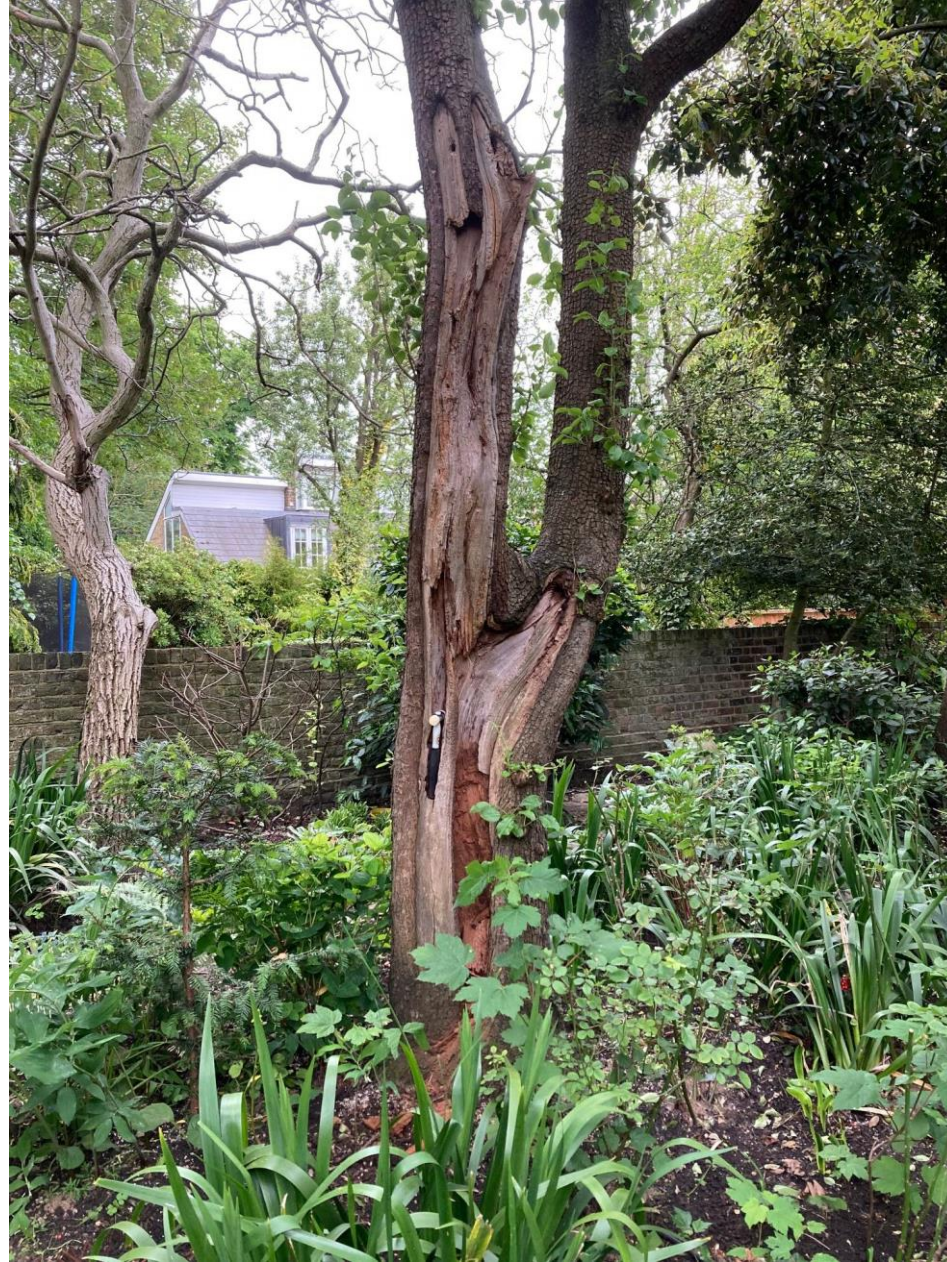
Photo no. 1 to show the old suspected bonfire scar on the common pear T2 Sounding Hammer included for scale Please note the dead walnut T1 behind T2
