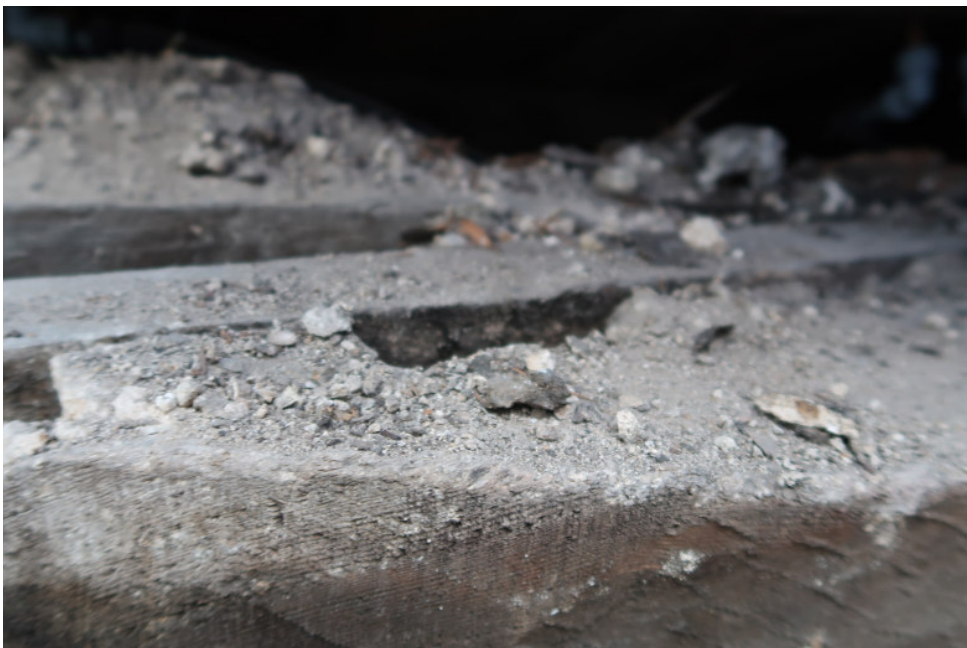
The three timbers don't appear to be connected.
