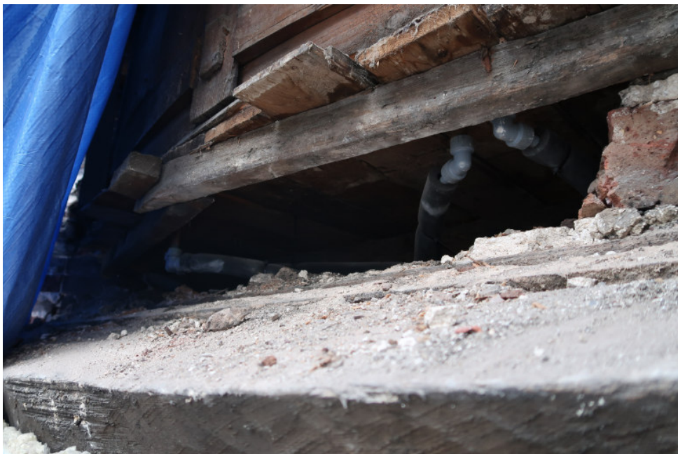
Dropped timber at front, floor timber over.
