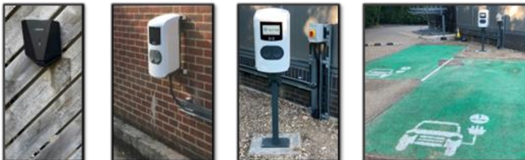
Figure 4-1 – Typical UK Power Networks EVCP Installations
