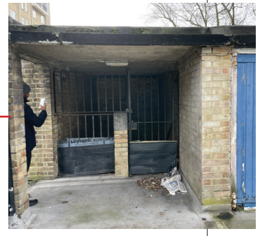
Existing iron metal gate leading to stair down into the space from the upper ground floor garages
