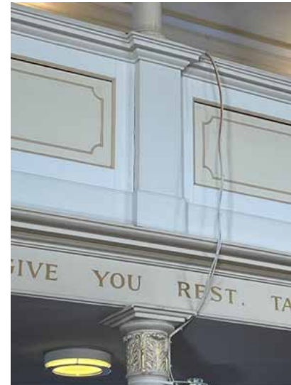
Images 14 and 15 - Item C Current loose cables hanging over the mezzanine balustrade, proposed to be neatly arranged.
