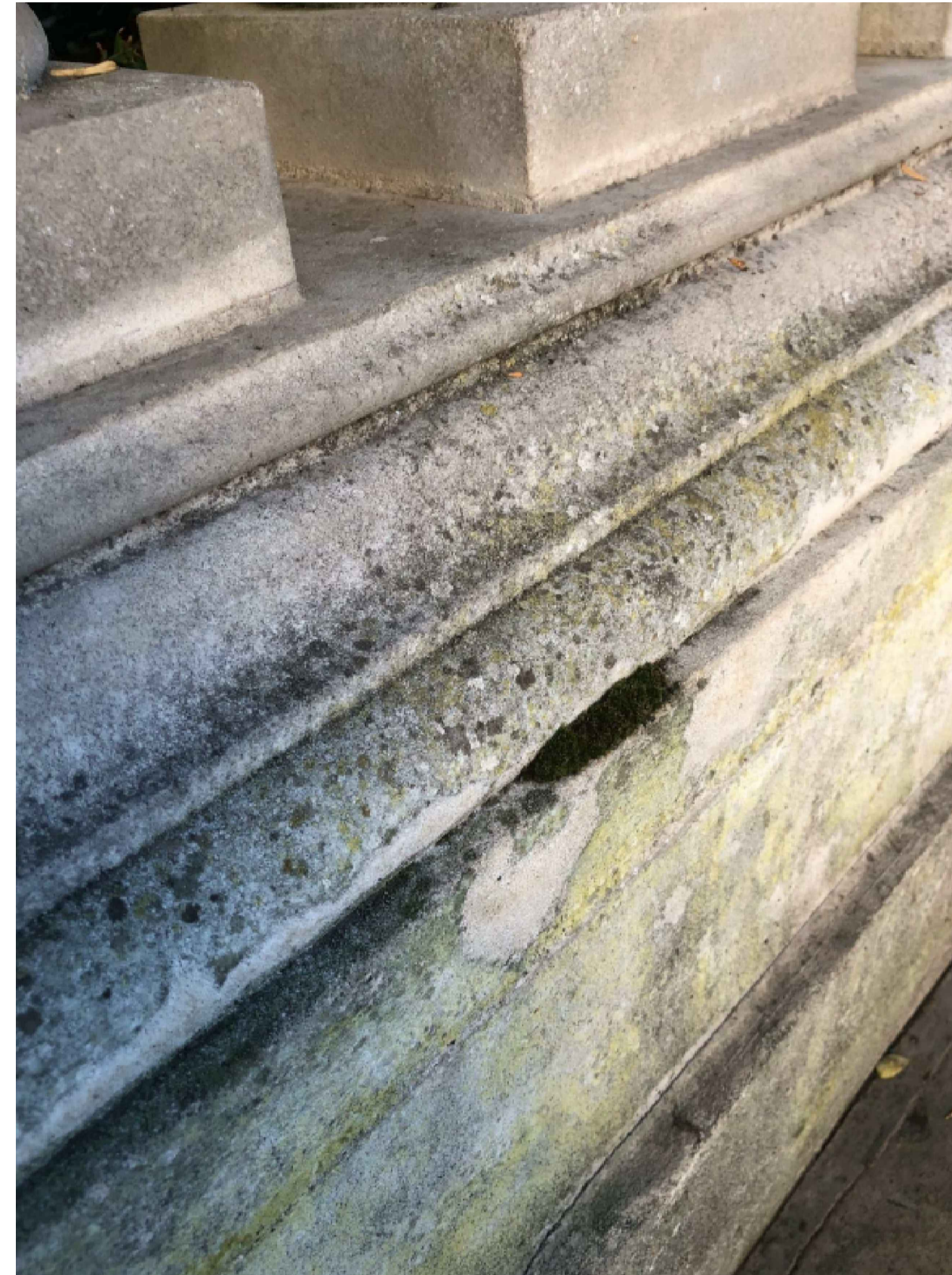
PHOTO SHOWING PLINTH PROFILE TO BE MATCHED ON CHESTER TERRACE
