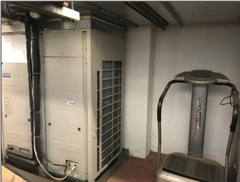
Mechanical Plant Room Basement 7 -15 Whitfield Street development
