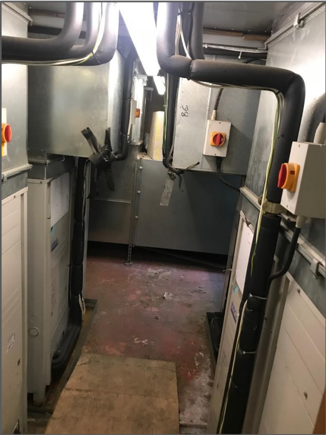
Mechanical Plant Room No 2 Basement 7 -15 Whitfield Street development
