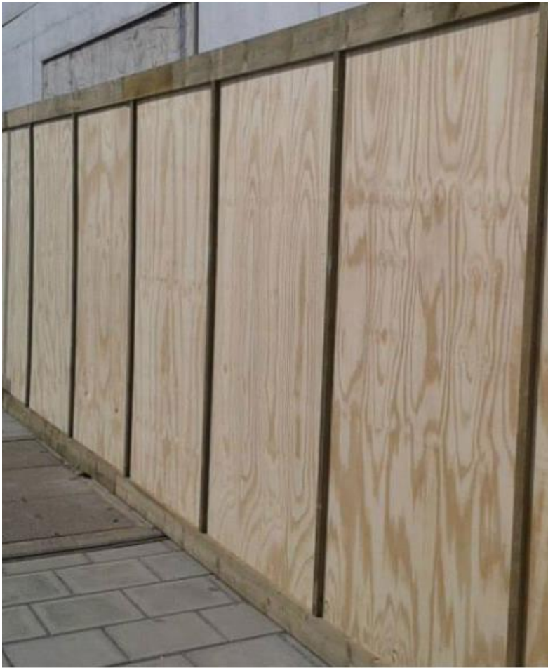
Example of stem protection for T4. Hardwood plywood sheet attached to wooden frame and fixed to floor using ground pins or similar.
