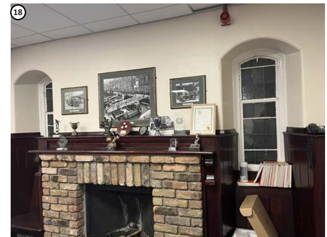
Plate 28 Historic windows to recreation room. High level penetrations would occur above and adjacent to these elements and would not affect any fixtures or fittings of interest.
