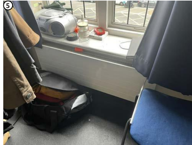
Plate 52 Penetrations for existing pipe work to radiators to be reused where feasible.
