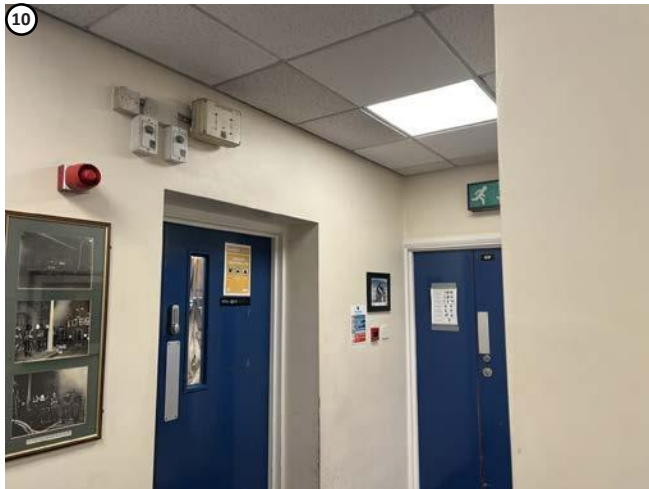
Plate 20 Left wall likely to be historic, penetration for heating pipes will occur to wall to right, which is later fabric.
