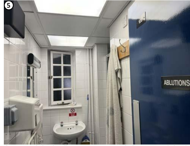
Plate 37 High level wall penetrations required above suspended ceiling would not affect significance of building.
