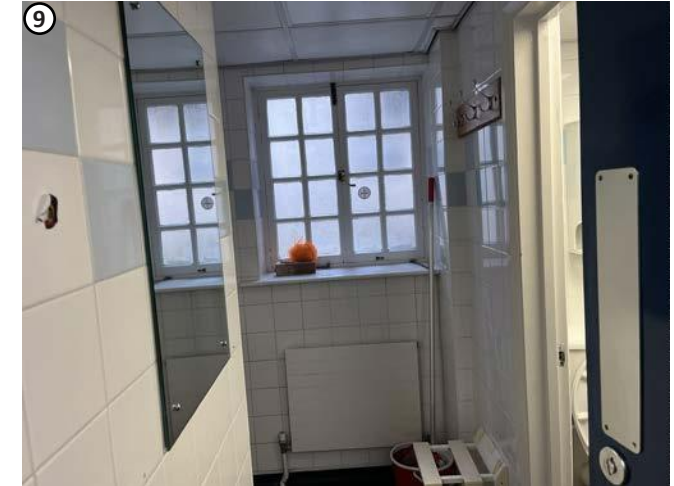
Plate 41 High level penetration required above suspended ceiling would not affect any fabric of interest.
