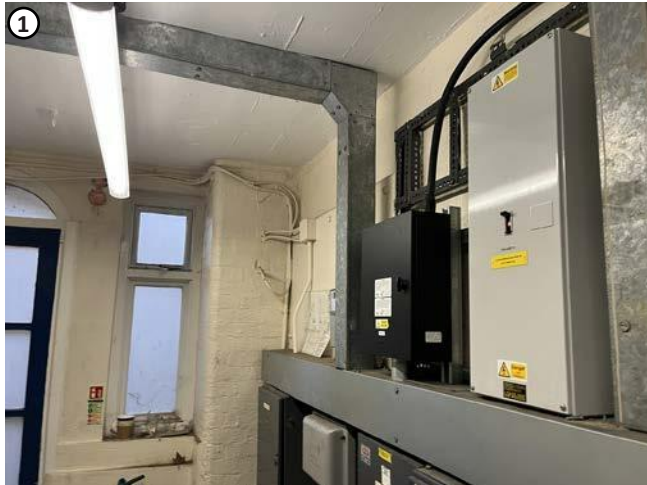
Plate 3 Showing no fabric of interest, a new cable tray will be installed here and small slab opening.
