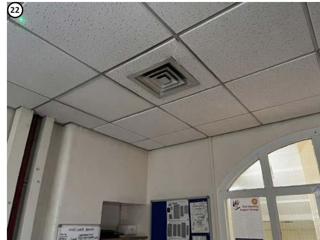
Plate 32 Station Manager's room, penetration required above suspended ceiling would not affect any fixtures or fittings of interest.
