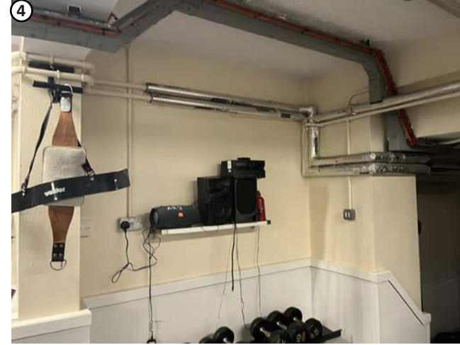
Plate 6 A small opening will be made 100mm from the top of the ceiling through the wall for heating pipes, helping to tidy up the cluttered pipe work.
