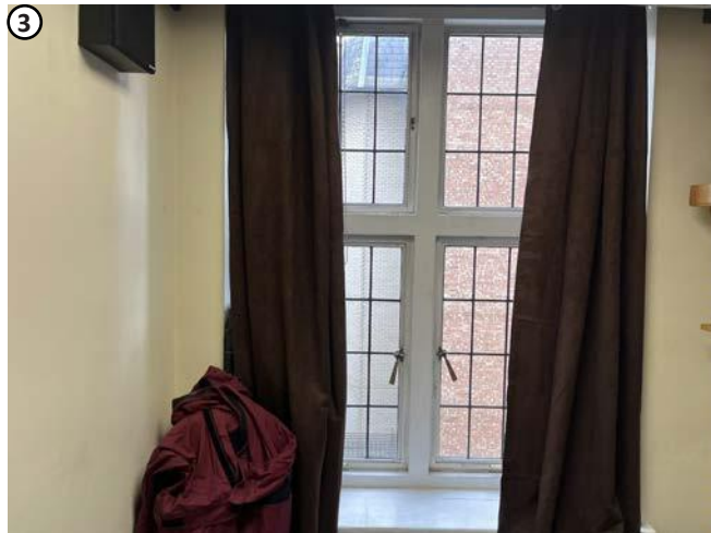
Plate 61 High level penetrations required above suspended ceiling would not affect any fabric of interest.
