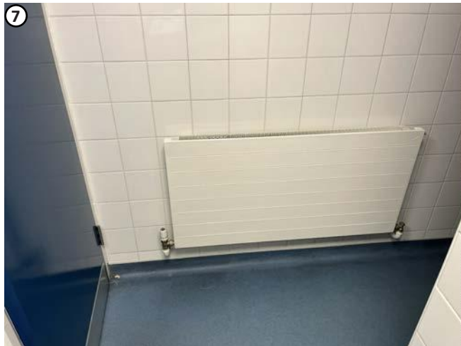
Plate 65 Showing modern bathroom of no interest. High level penetrations required above suspended ceiling would not affect any fabric of interest.
