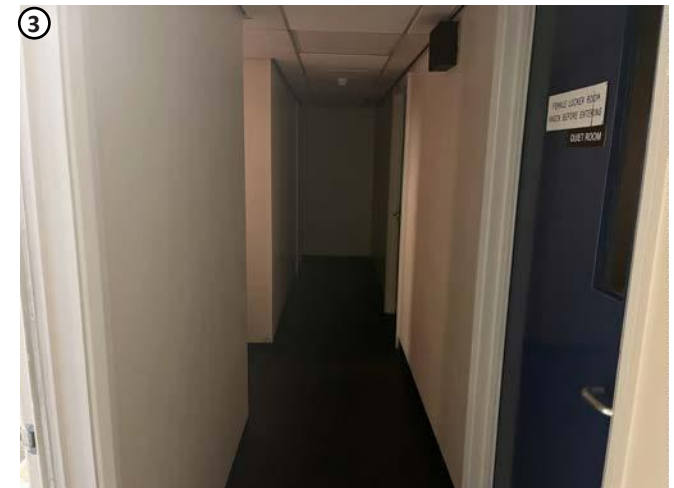
Plate 50 High level penetrations required above suspended ceiling would not affect any fabric of interest.
