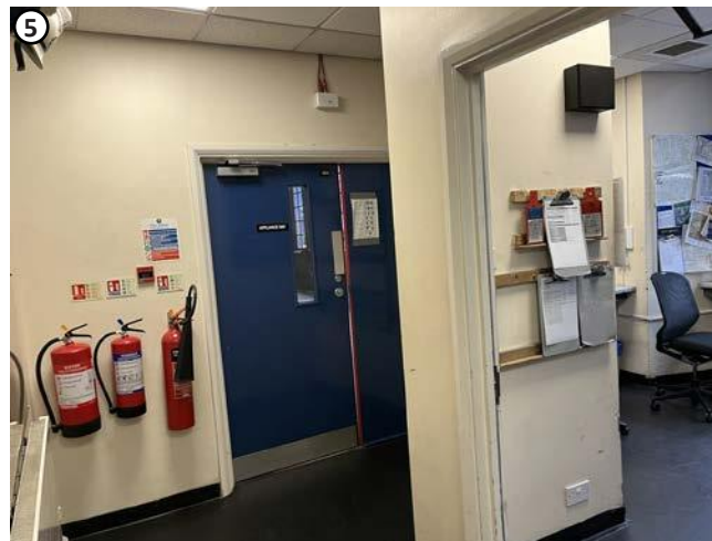
Plate 15 Showing modern fabric installed in previous engine room. High level wall penetration would be hidden in suspended ceiling.
