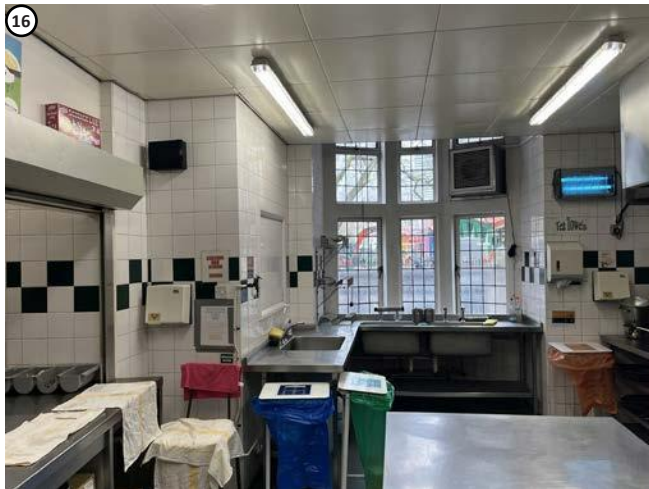
Plate 26 View of kitchen, openings to slab required to right and above ceiling to left. Potential for some load bearing walls to be affected, but would not affect significance.
