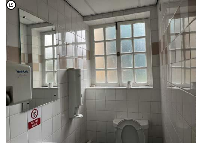
Plate 47 High level penetrations required above suspended ceiling would not affect any fabric of interest.
