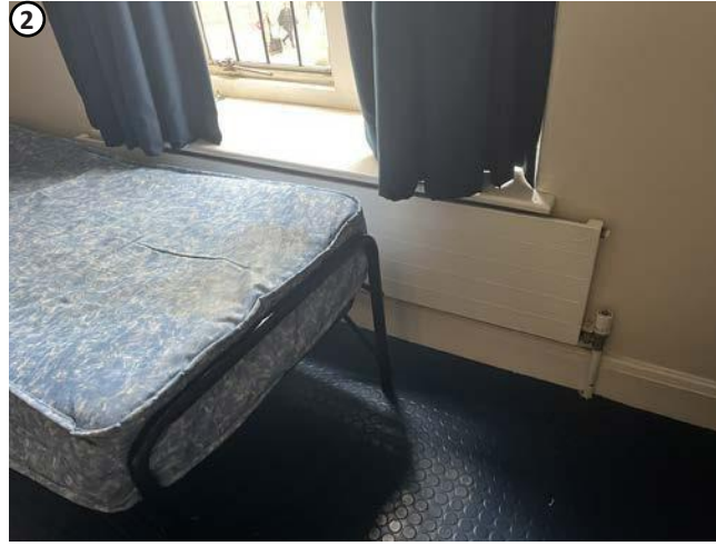
Plate 34 Penetrations for existing pipe work to radiator to be reused where feasible.
