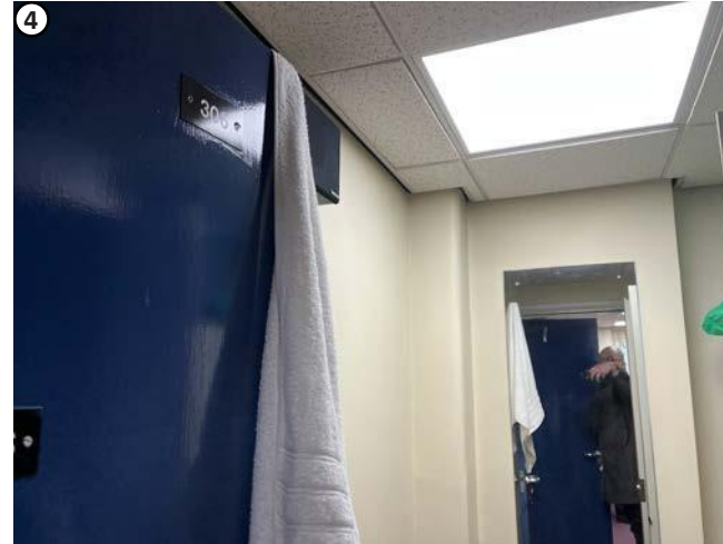
Plate 62 High level penetrations required above suspended ceiling would not affect any fabric of interest.
