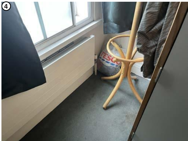
Plate 51 Penetrations for existing pipe work to radiators to be reused where feasible.
