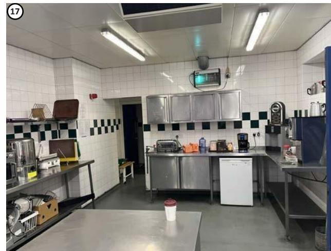
Plate 27 Slab penetration needed to top left corner above suspended ceiling. Would not affect significance.
