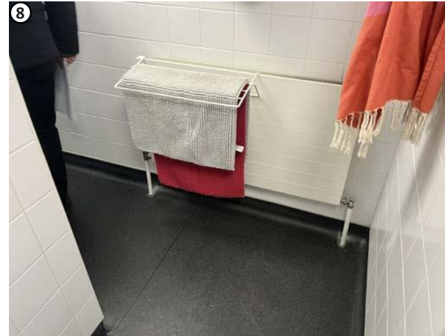
Plate 56 Penetrations for existing pipe work to radiators to be reused where feasible.
