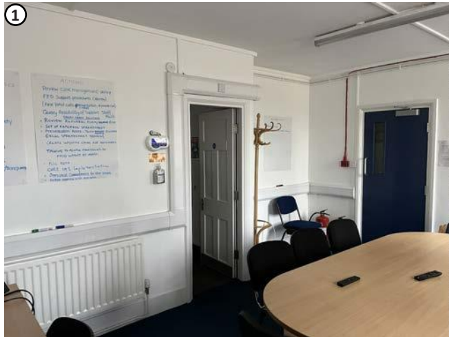
Plate 59 General view showing condition of this floor with most original features removed. Some original fireplaces do survive, works to this level are confined to the room through the central door.
