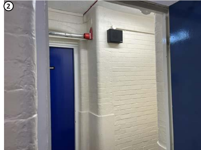
Plate 4 A small opening will be provided beneath ceiling level for hot water pipes.
