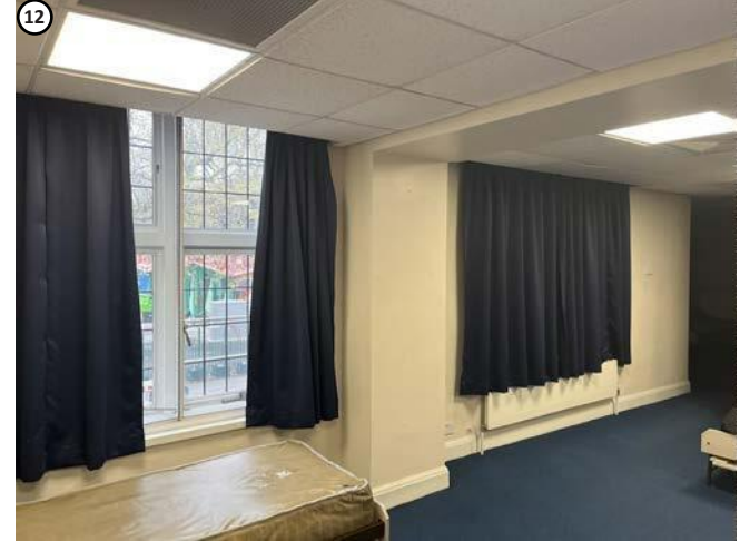
Plate 44 High level penetration required above suspended ceiling would not affect any fabric of interest.
