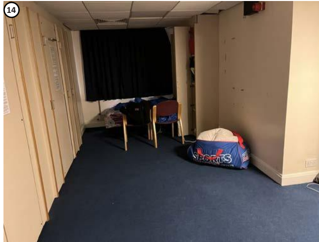
Plate 46 High level penetration required above suspended ceiling would not affect any fabric of interest.
