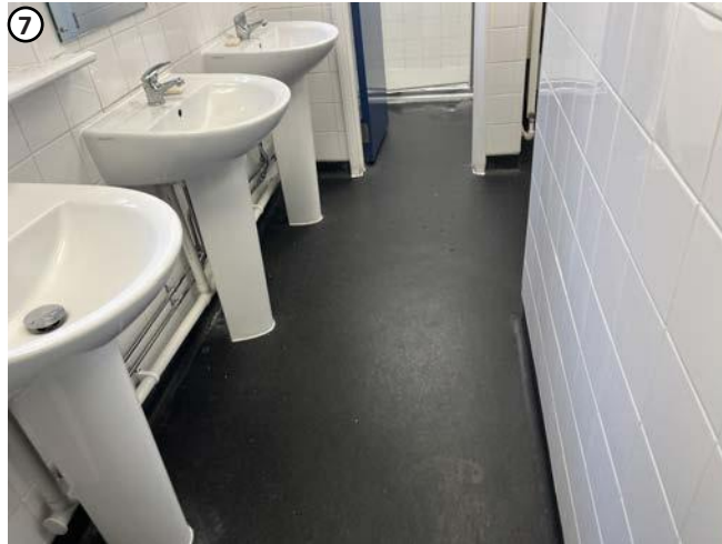
Plate 55 Modern toilets of no interest. High level penetrations required above suspended ceiling would not affect any fabric of interest.
