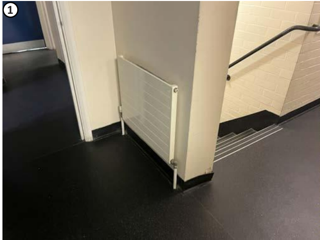
Plate 48 Penetrations for existing pipe work to radiators to be reused where feasible.
