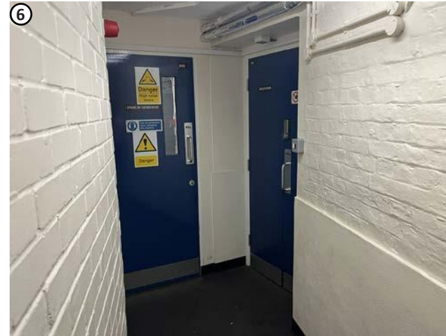
Plate 8 New heating pipes will be located at high level here.
