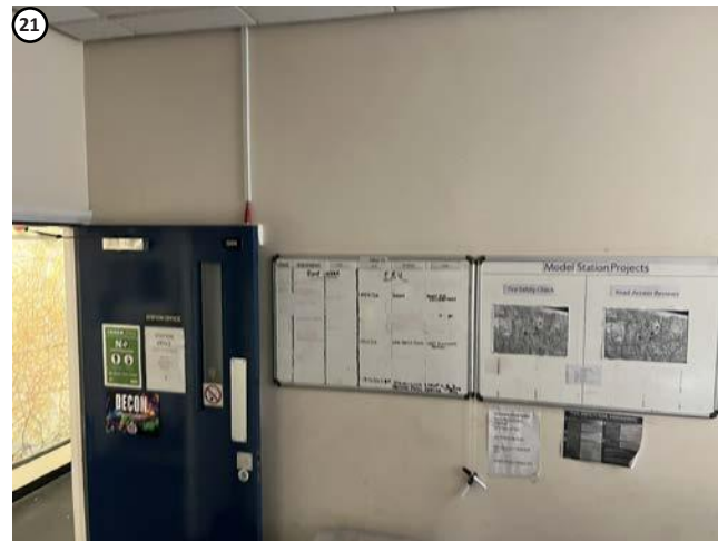
Plate 31 Station Manager's room, penetration required above suspended ceiling would not affect any fixtures or fittings of interest.
