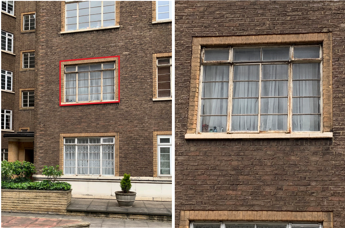
Context view of the window concerned, highlighted in red Detail showing the poor condition of the window
