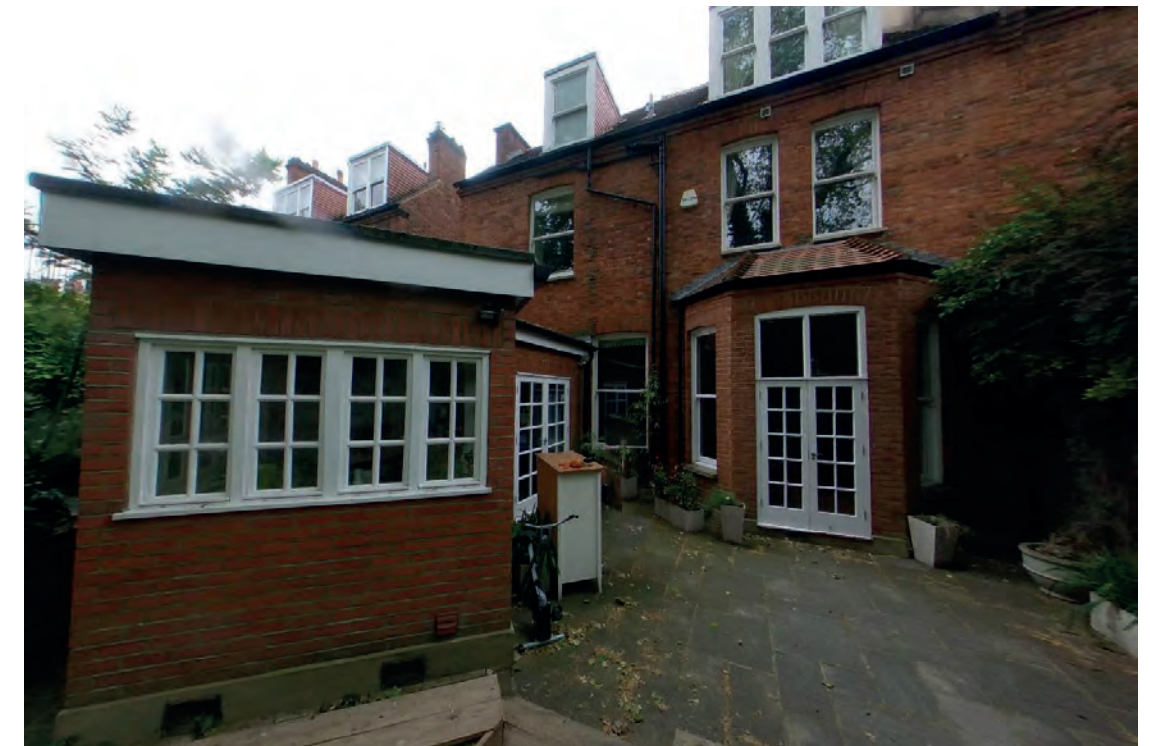
Existing rear facade is relatively orderly, lacking the ornamentation of the front facade
