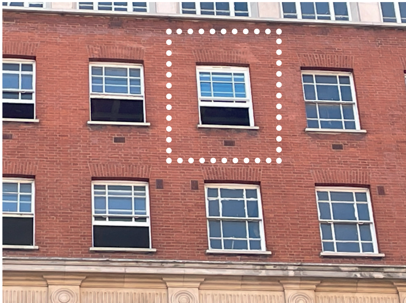
Fig. 12. Mock-up sash window, front elevation. (Please note this does not feature the proposed acoustic attenuator. This is shown on drawing AA(31)001.)
