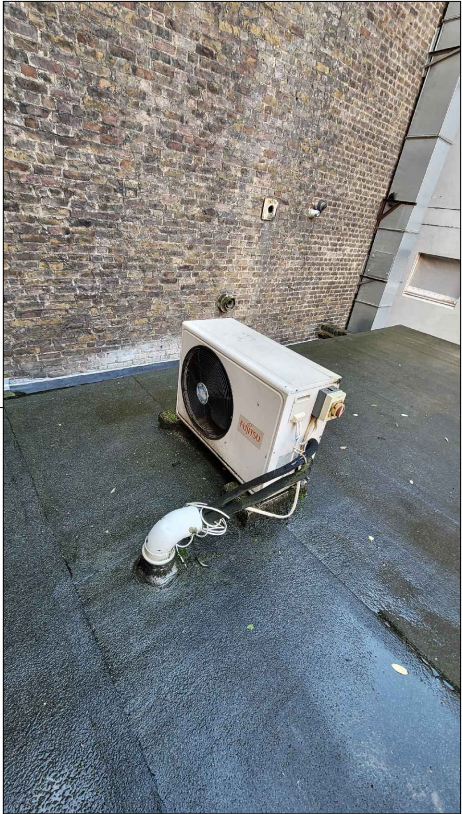
PRE EXISTING AC OUTDOOR UNIT
