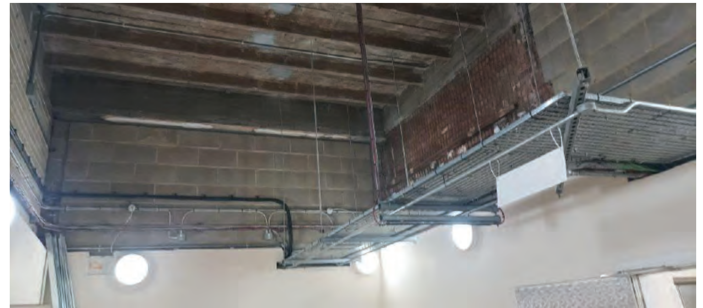
Level B1 - North Stair - Landing ceiling. Showing current electrical containment.
