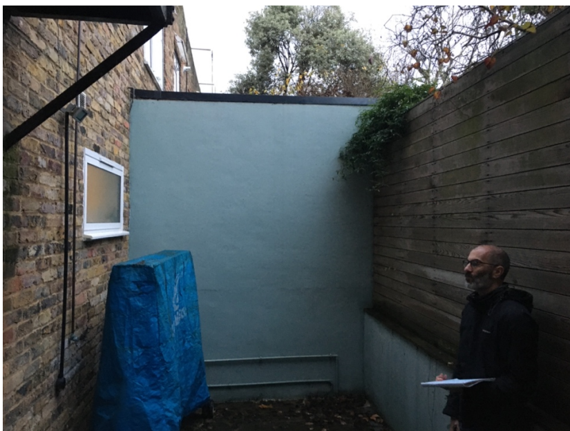
Wall to the rear of the property on the south-west side (no.31)
