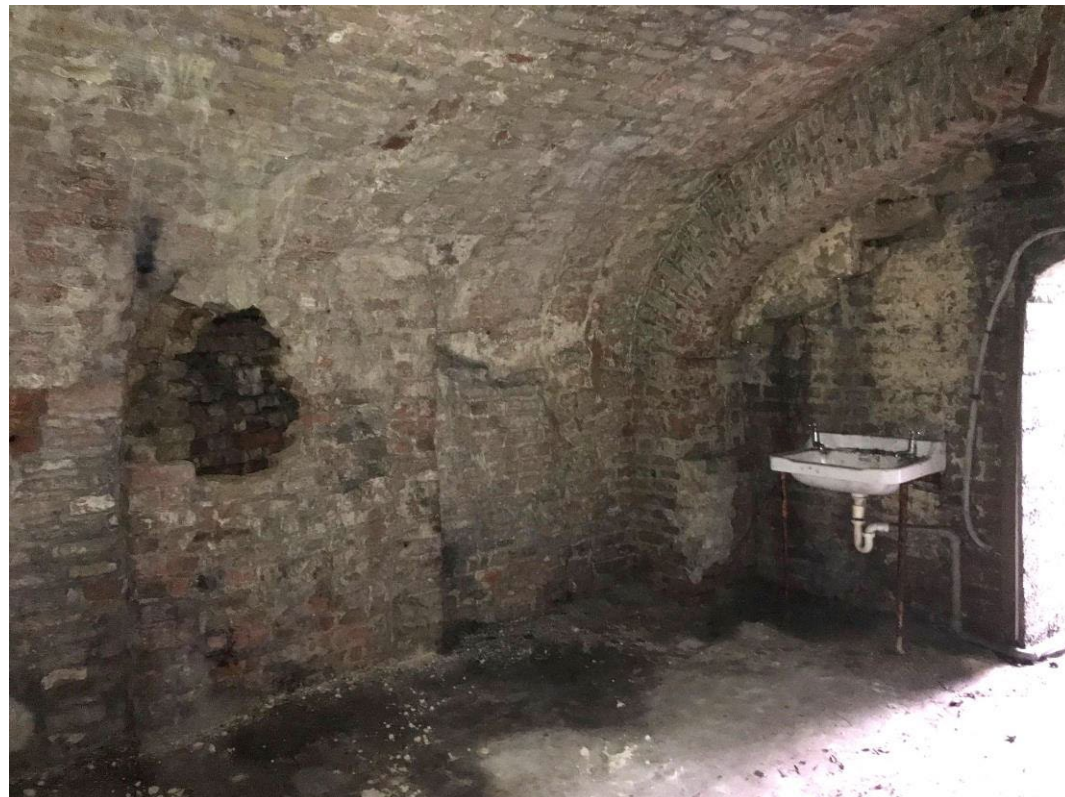
Plate 24: Internal part of vault built into the Vault built into the Listed (Grade II) Garden Walls, Terraces and Steps of Numbers 1-6 and Garden Arbour to Number 6 (1378982). This is located below the steps from the upper to the lower back garden.
