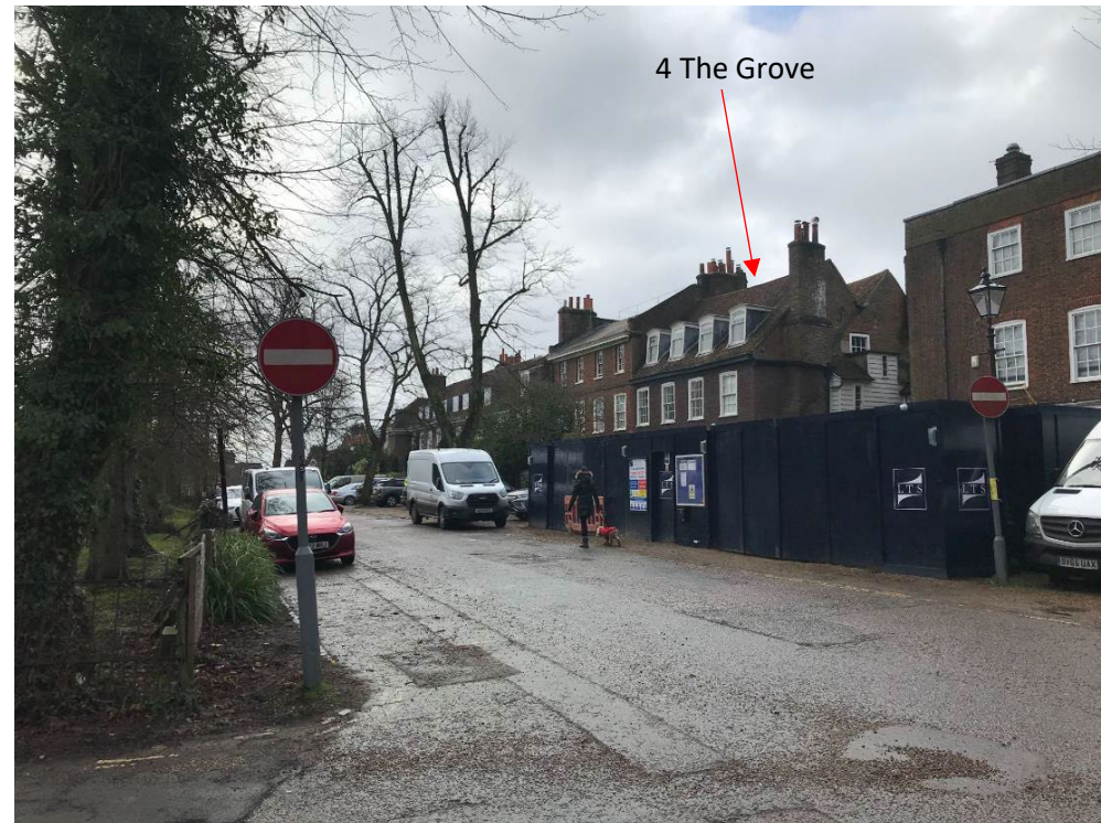
Plate 6: Photograph taken from The Grove, facing the front of 4 The Grove . The blue hoarding is outside No. 5 in which a large basement is currently being excavated in the front garden.
