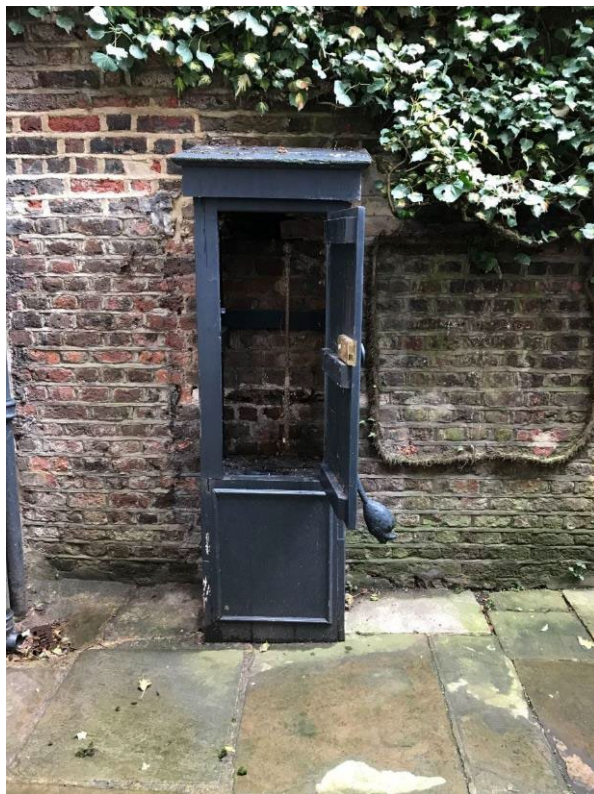
Plate 12: In-situ water pump with machinery still present (lower ground floor external)
