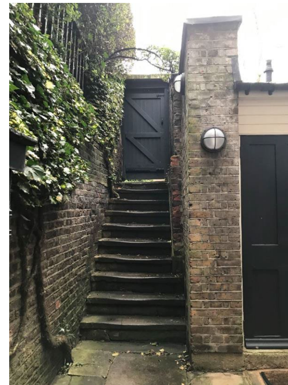
Plate 11: Steps down to the lower ground floor area (external). The steps lead down from the front garden.
