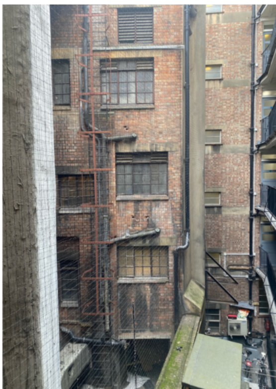
Figure 4 (above): View of the lightwell area from first floor level including external access walkways of Phoenix House to the right
