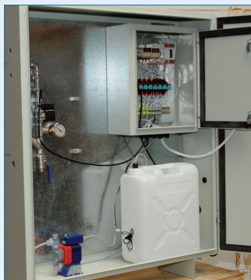
INTERIOR OF AUTOWASH CABINET
