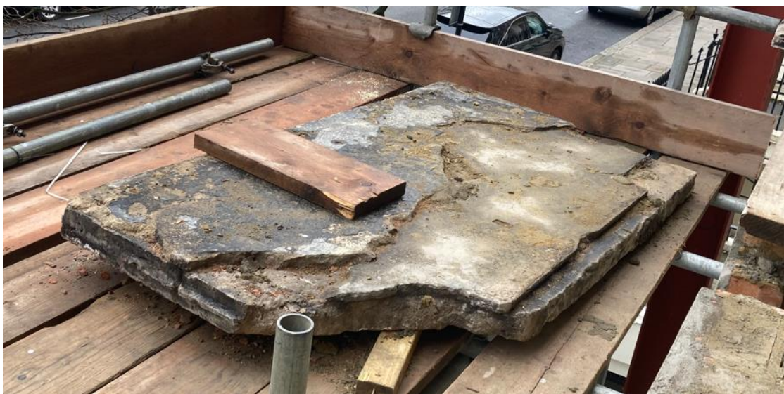
Figure 3 - the extent of damage to the stone slabs.
