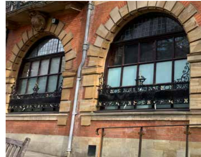
Figure 5.1 2021 Photograph of the building's ground floor windows with sign boards retained in-situ. The sign boards display no signs and screws and fixings are visible
