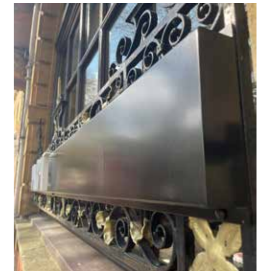
Figure 5.4 The signs are fixed to existing sign boards and their installation avoided interference with the historic railings and windows
