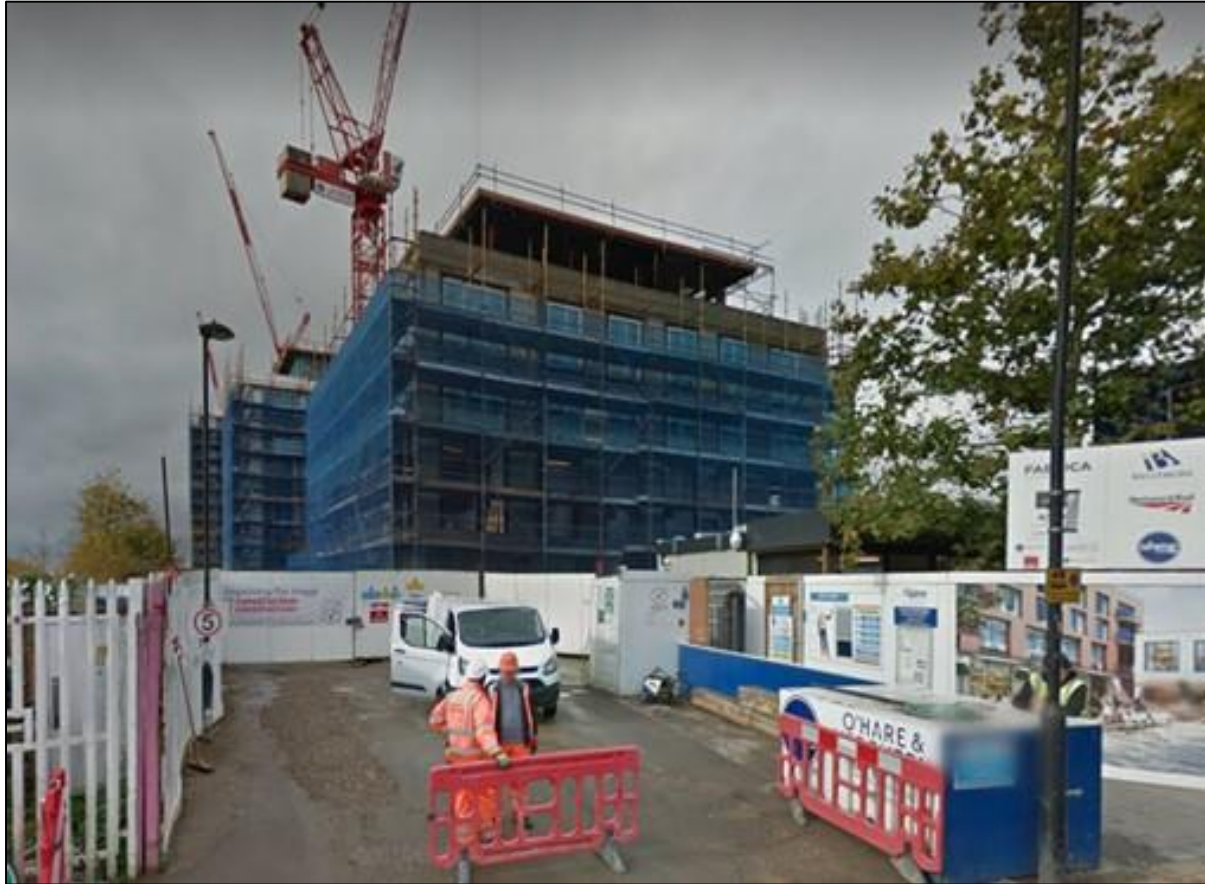
Fig. 4: Example of negative visual impact of scaffolding and generic sheeting on the street scene at West Hampstead Square, London
