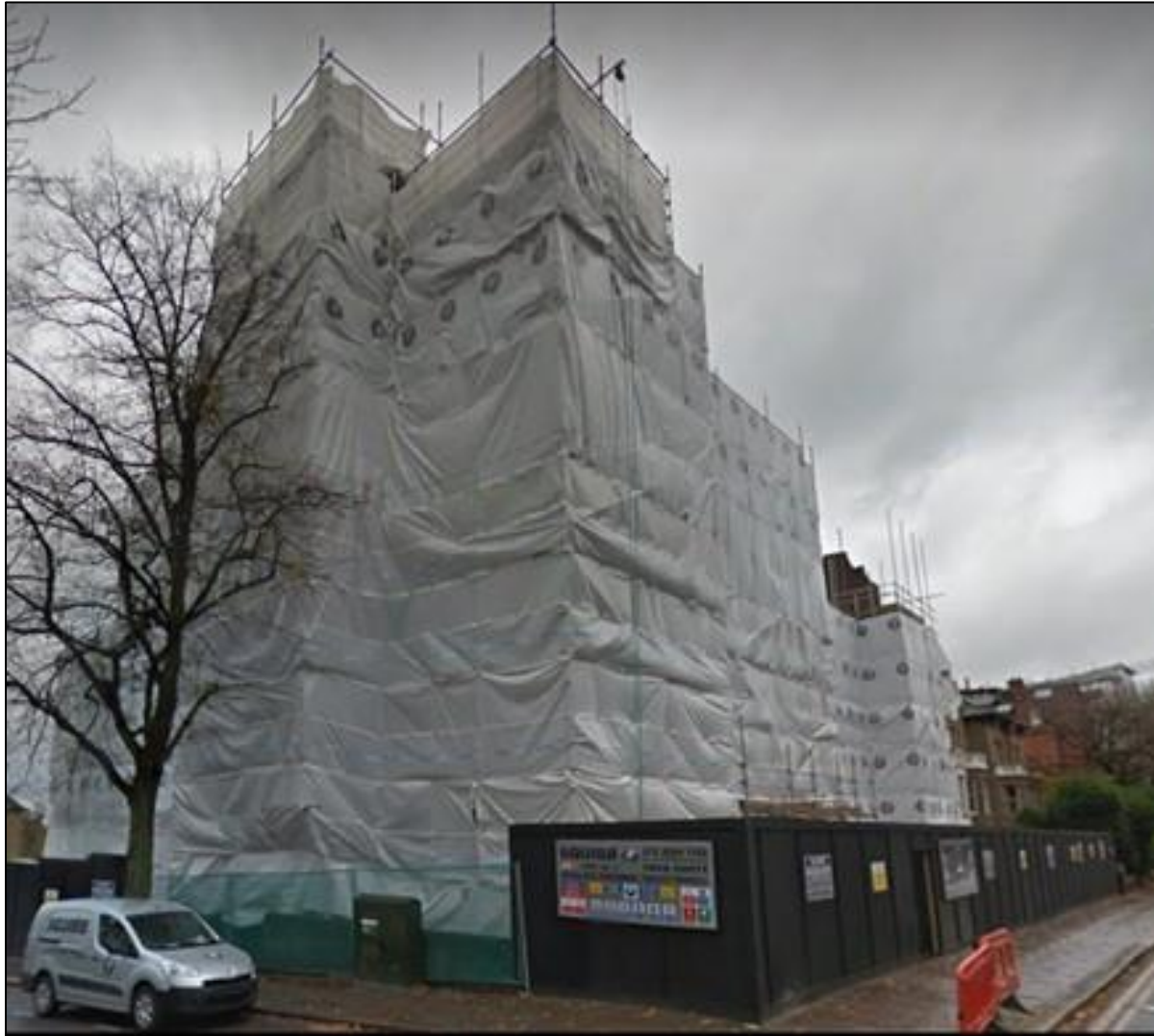
Fig. 1: Example of negative visual impact of scaffolding and generic sheeting on the street scene at 79 Fitzjohn's Ave, London
