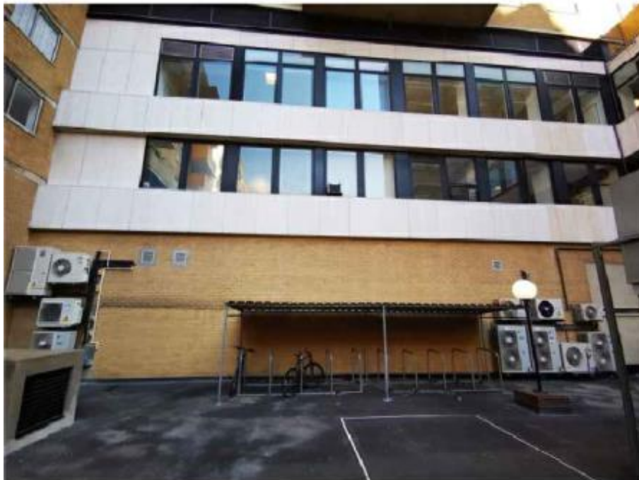
EXISTING OUTDOOR A/C UNITS
