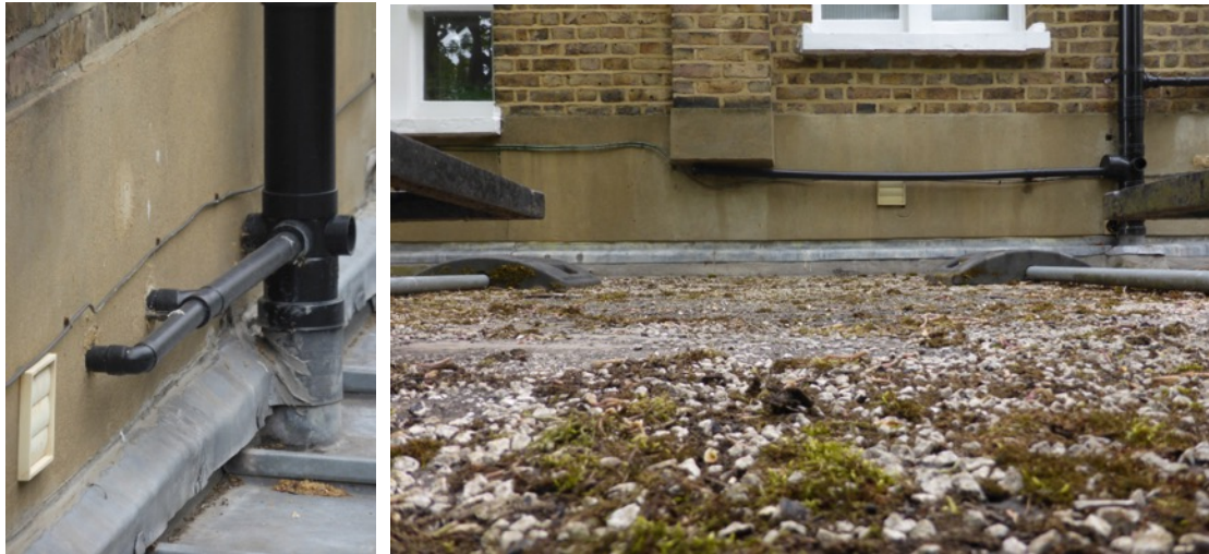
Figs. 35,36 Locations for external intake and exhaust grilles on the South and West ranges
