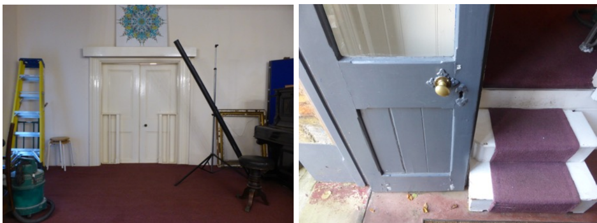
Figs. 10,11 doors to the current Library, unsafe stage steps next to courtyard entrance door
