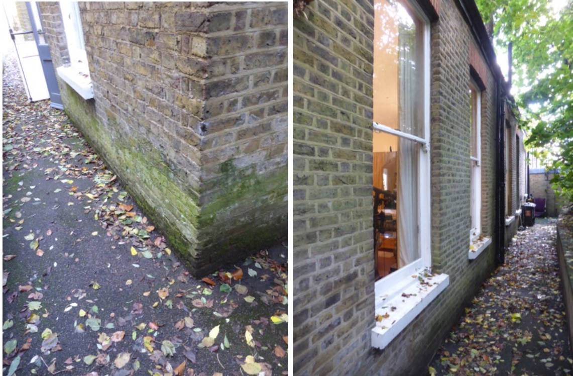
Figs. 22,23 Water damage to the Hall walls, raised external ground level
