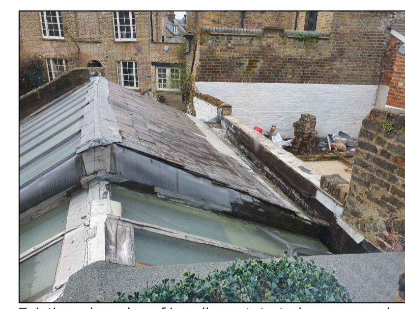
Existing glazed roof in adhoc state to be removed and replaced with new glazed roof
