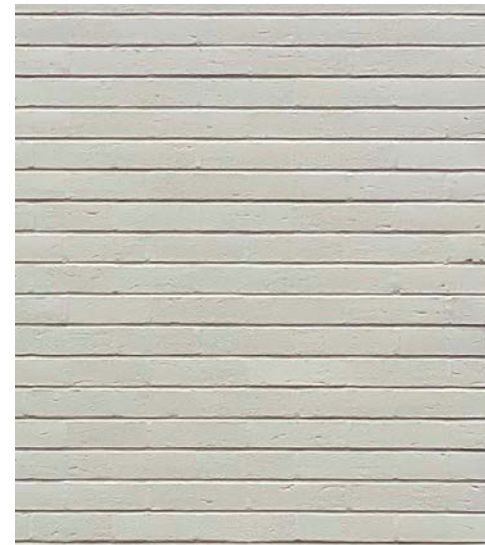
White painted brickwork with raked out horizontal joints and flush perpend to match existing.
