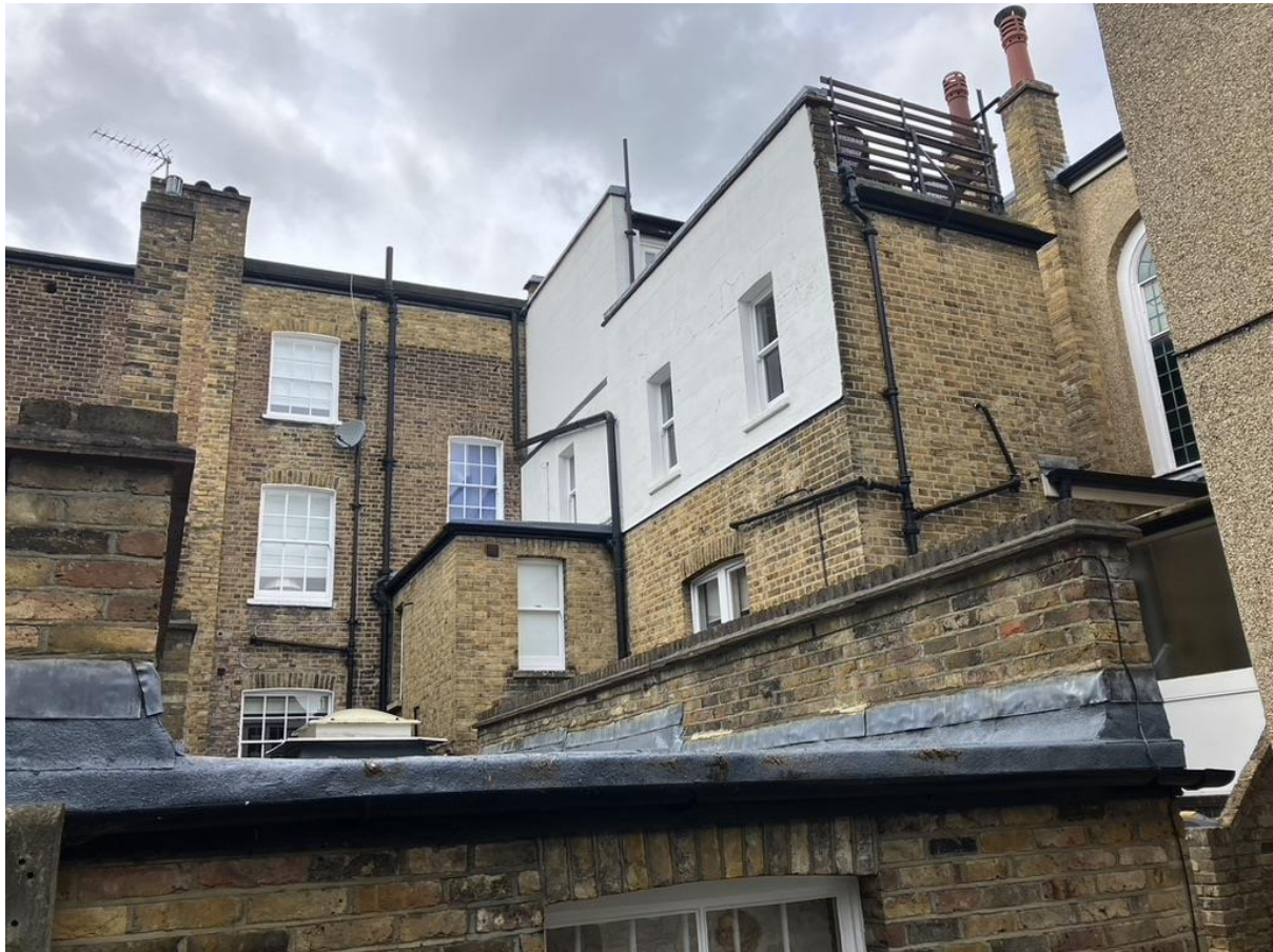
Rear elevations to nos. 3 (left) and 4 (right) Holly Place showing additions of 1912-13 (right) and 1971 (foreground)
